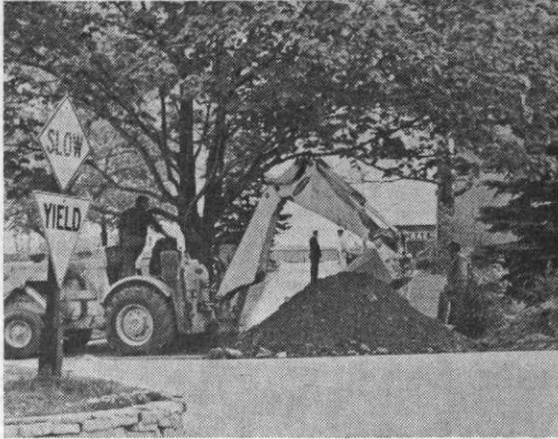
Maintenance men prepare to make a new walk in area by Meagher Hall.
