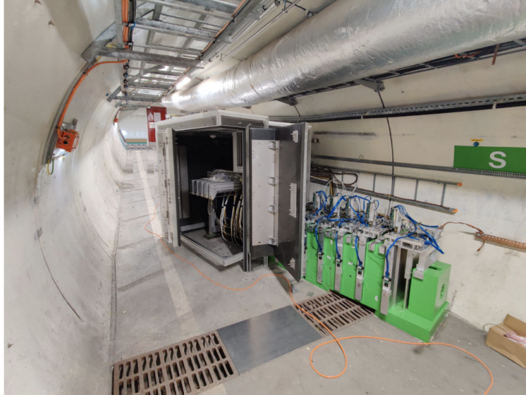
Figure 51: Global view of the detector in TI18 after the installation of the neutron shield.
