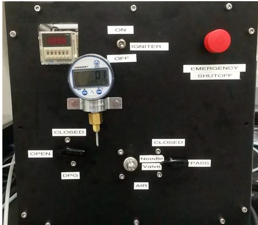
Figure 4.7: Front of the Control Panel.
