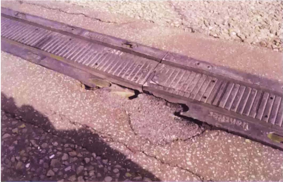
Figure 2-2 Damaged bridge joint
