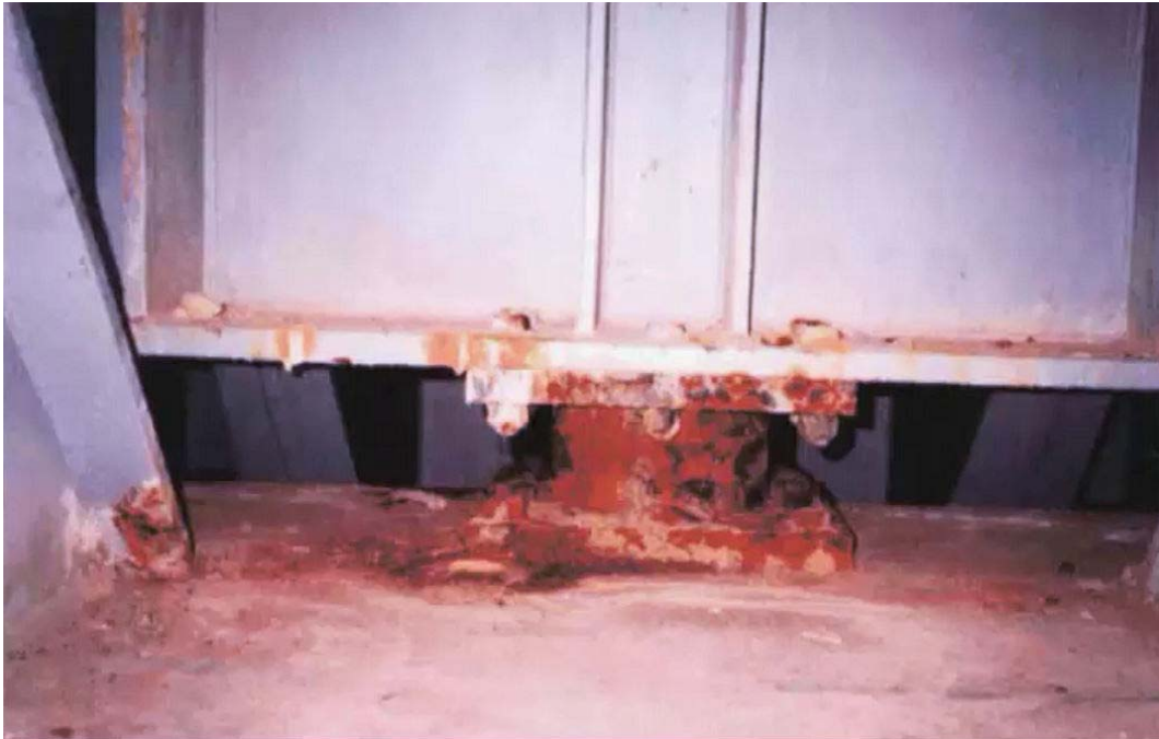
Figure 2-3 Corroded bridge bearing
