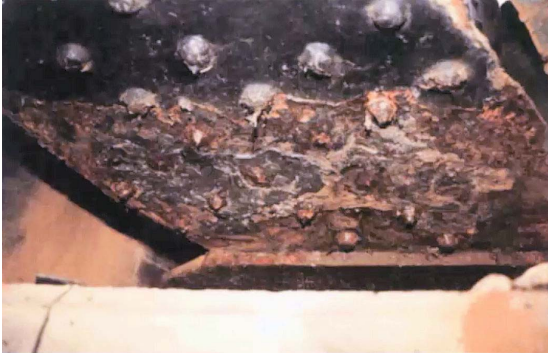
Figure 2-4 Corroded bridge girder
