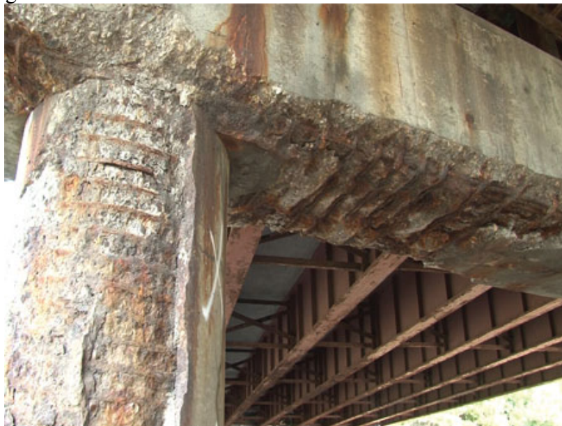
Figure 2-1 Bridge bent damaged by a leaking expansion joint
