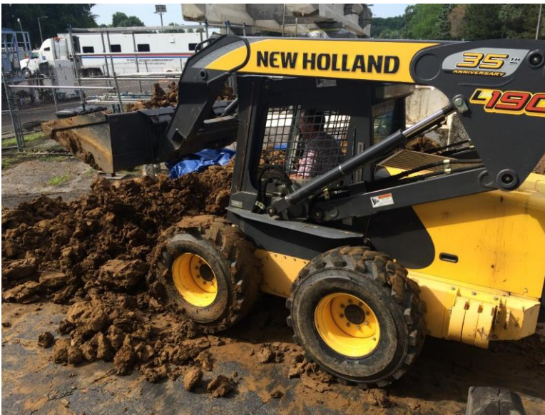
Figure 3.7. Use of skid-steer loader for breaking and spreading the HPC soil for further drying
