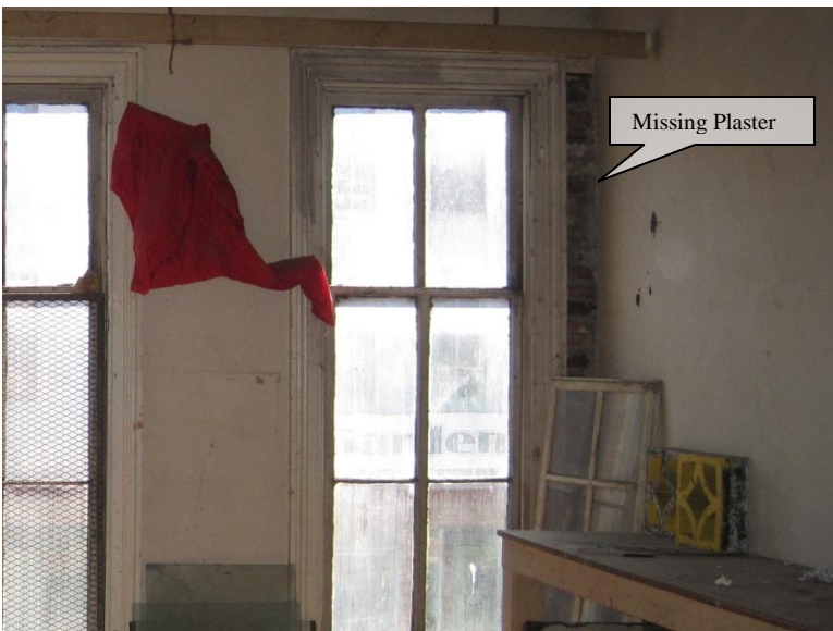
Figure 77. Second Floor: missing plaster on south wall.
