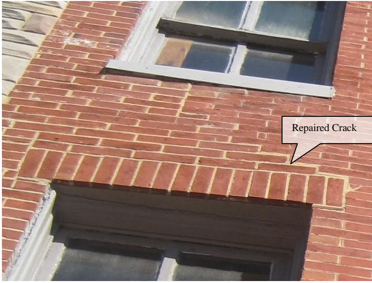
Figure 22. Exterior: second floor west lintel and repaired crack above.
