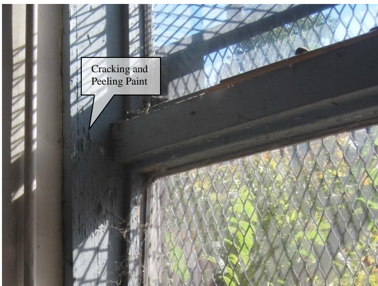
Figure 60. First Floor: cracking and peeling paint on storefront window frame.
