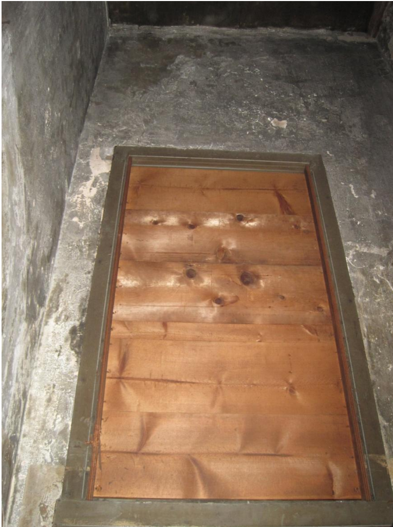
Figure 70. Second Stair Landing: window opening sealed with wood boards.
