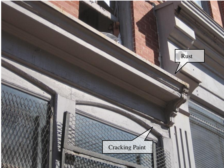
Figure 31. Exterior: cracking and peeling paint; rust on flashing.
