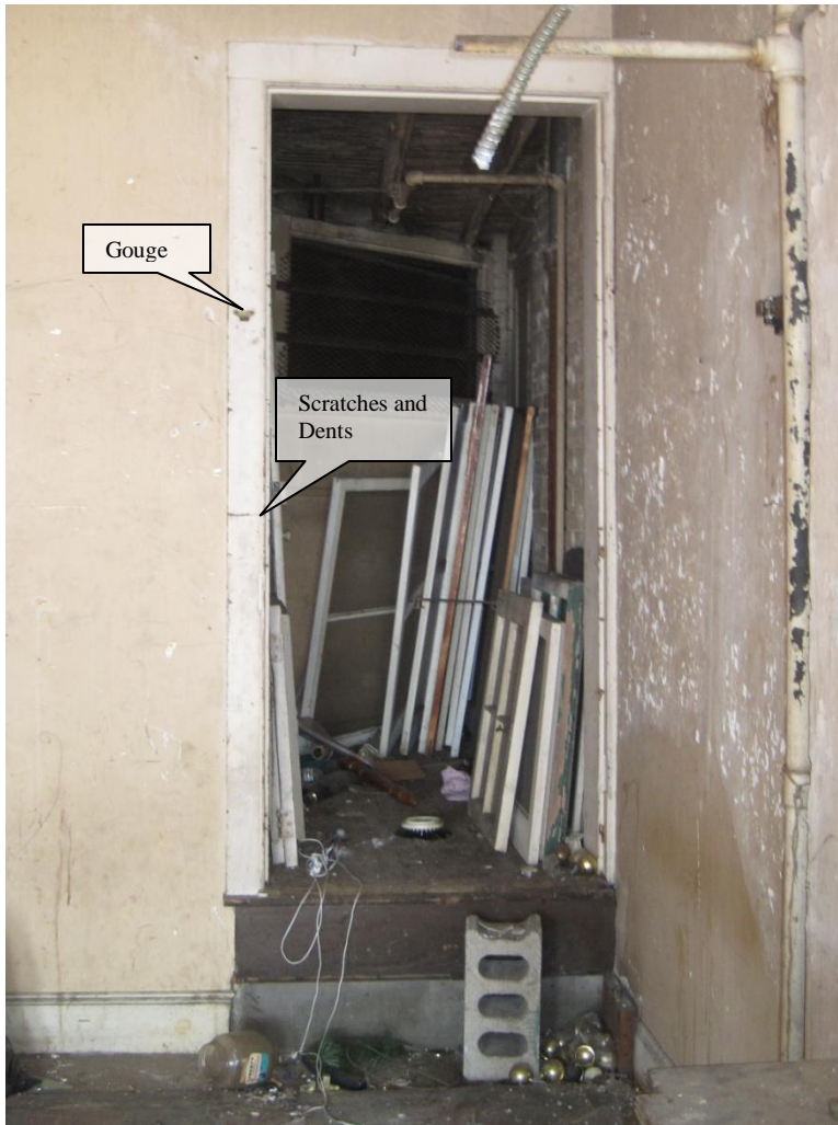
Figure 48. Second Floor: worn edges, scratches, and gouges in doorway trim.
