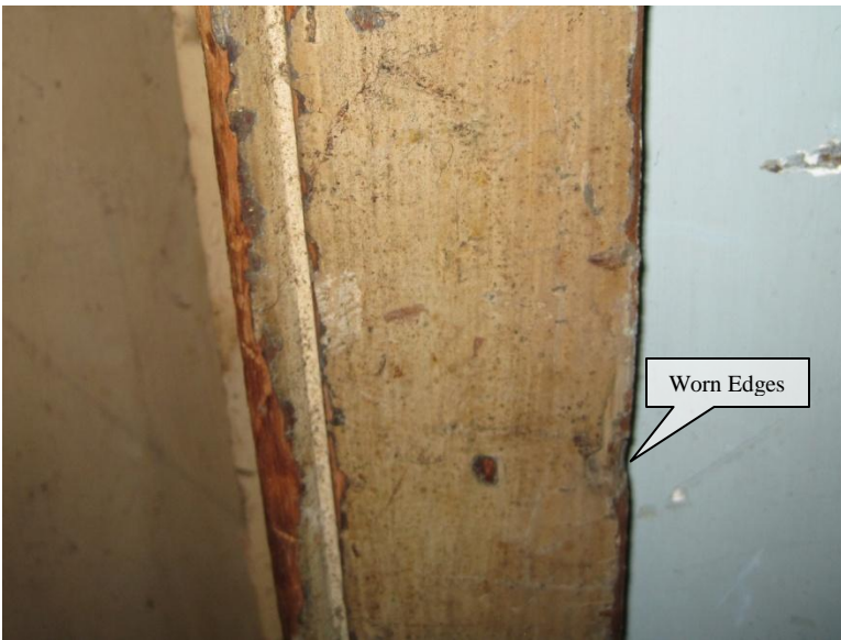
Figure 46. First Stair Landing: worn edges on window trim.
