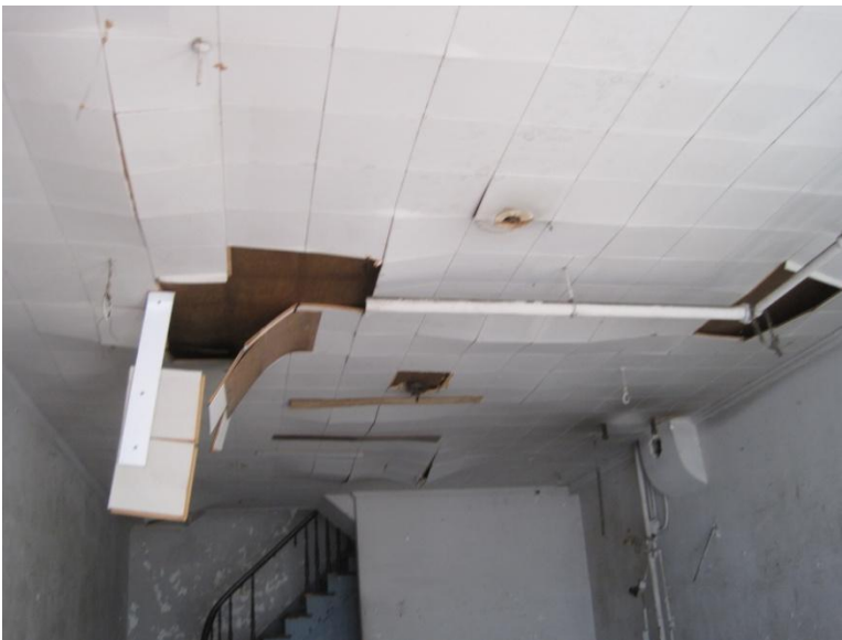
Figure 81. First Floor: ceiling tiles falling down.
