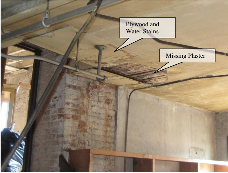
Figure 85. Third Floor: water damage and plywood patching.
