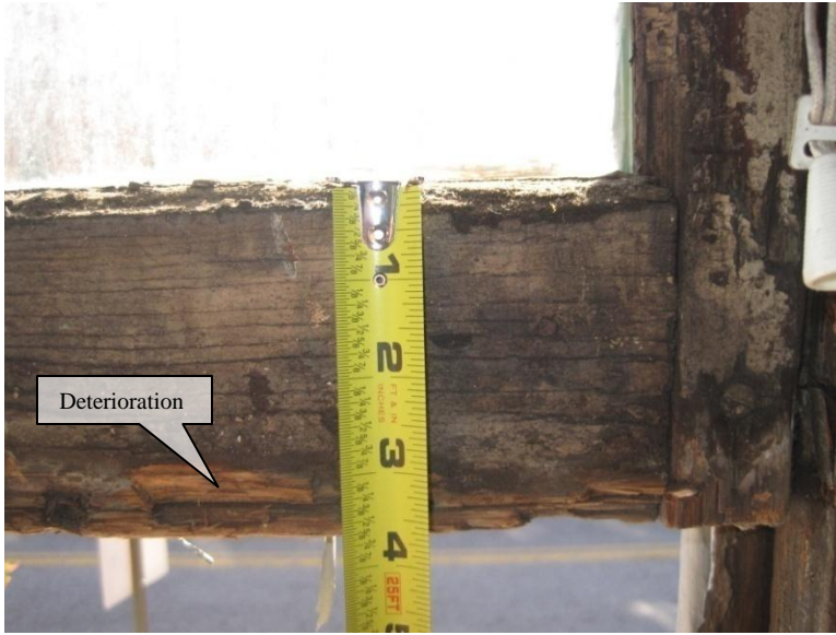
Figure 63. Second Floor: deteriorated bottom rail on east window sash.
