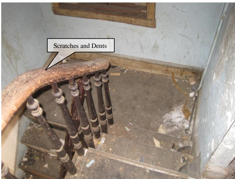
Figure 36. First Stair Landing: scratches and dents on handrail and balusters.
