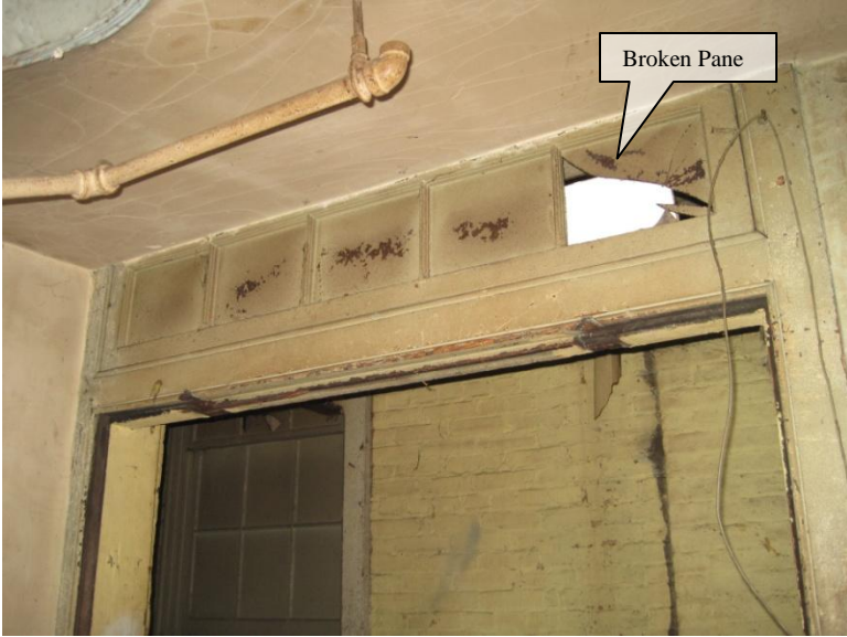
Figure 61. First Floor: painted glass and broken pane on doorway under stairs.
