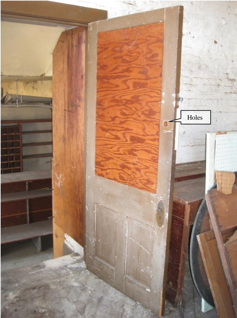
Figure 57. Third Floor: holes in stile and plywood in place of glass on connecting door.
