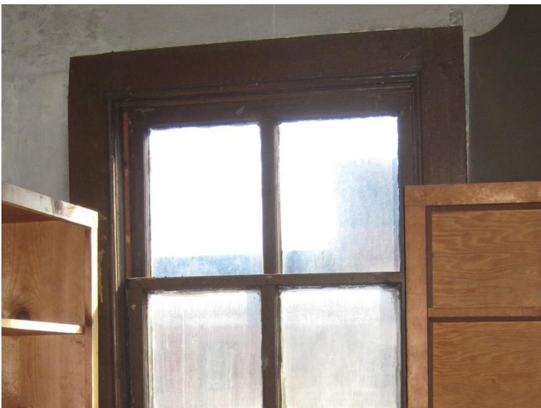
Figure 54. Third Floor: window trim with little wear.
