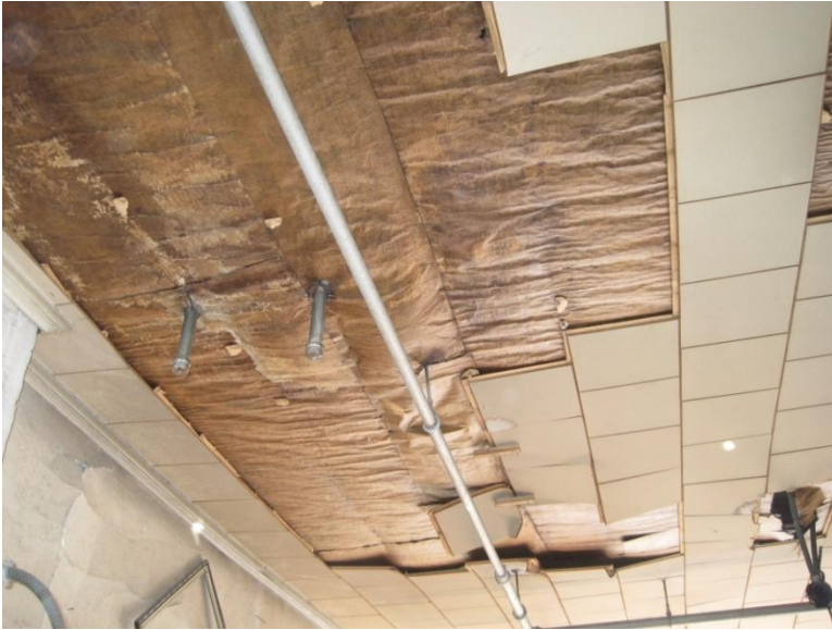
Figure 82. Second Floor: missing ceiling tiles.
