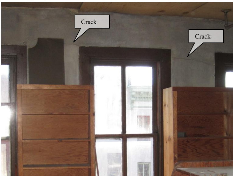
Figure 80. Third Floor: cracks in plaster on south wall.
