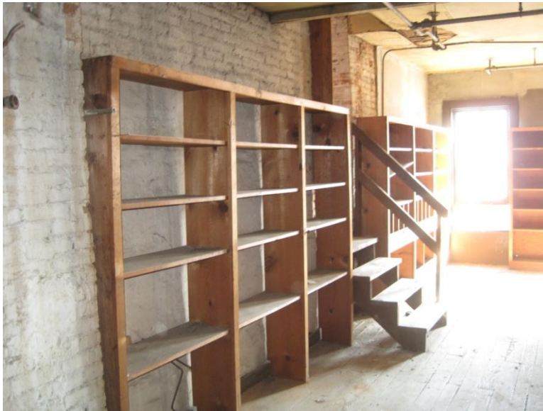
Figure 79. Third Floor: missing plaster on east wall.
