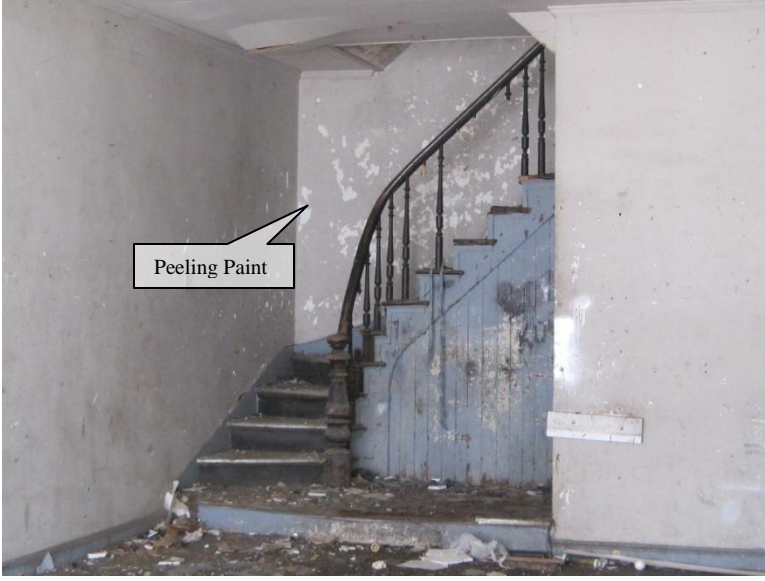
Figure 75. First Floor: peeling paint on north and west walls.
