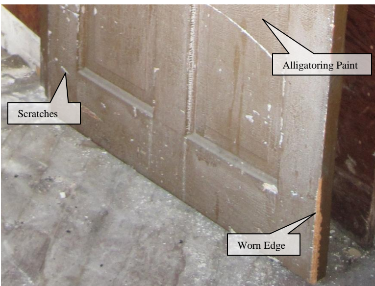
Figure 58. Third Floor: damage to stile edge, scratches in the surface, and alligatoring paint on connecting door.
