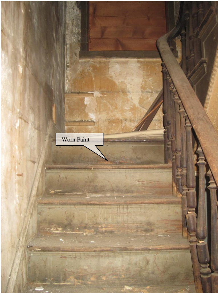
Figure 38. Second Floor: paint wearing away on both treads and risers.
