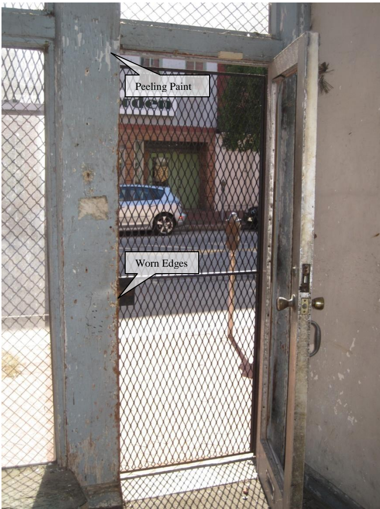
Figure 44. First Floor: peeling paint and wear at corner edges on south wall trim.
