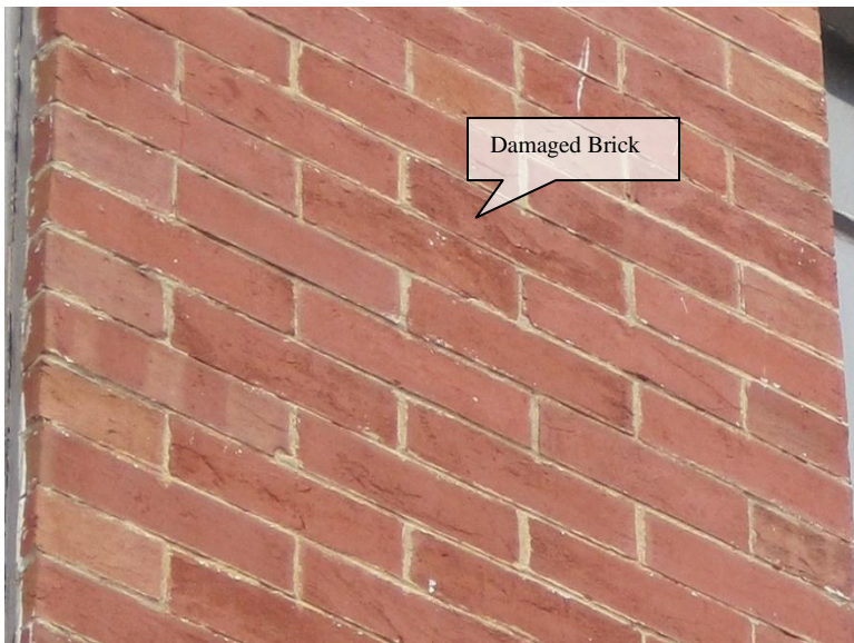
Figure 21. Exterior: damaged brick surface.
