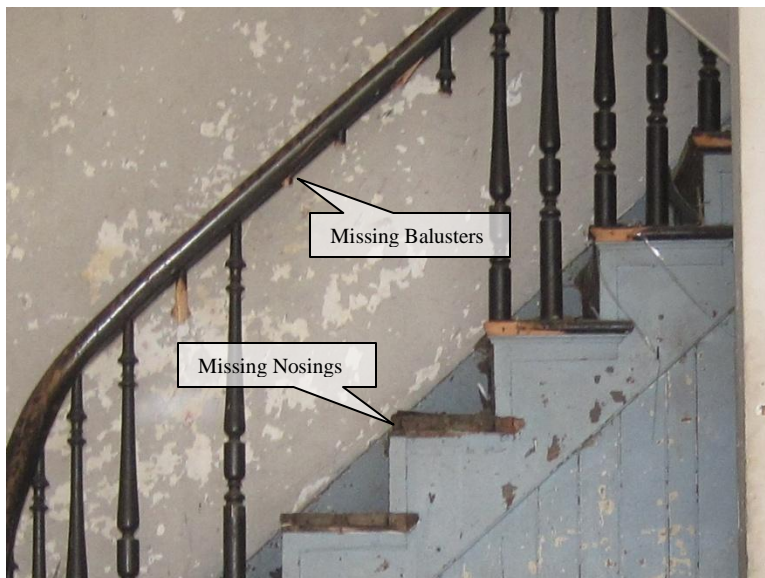
Figure 34. First Floor: missing balusters and nosings.
