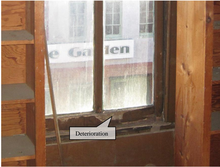
Figure 66. Third Floor: deteriorated bottom rail of sash on middle window.
