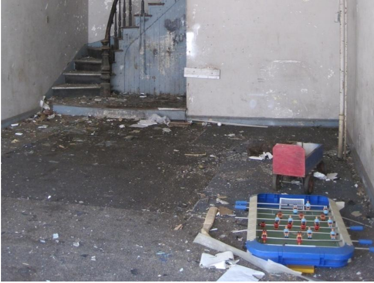
Figure 71. First Floor: worn carpeting.
