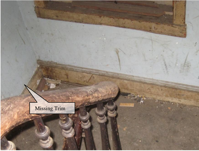
Figure 45. First Stair Landing: missing baseboard piece and damaged window trim.
