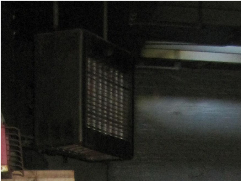
Figure 90. First Floor: existing unit heater located in larger building directly behind 1428.
