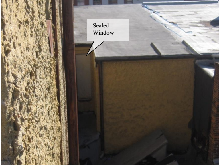
Figure 69. Exterior: sealed third floor north window.
