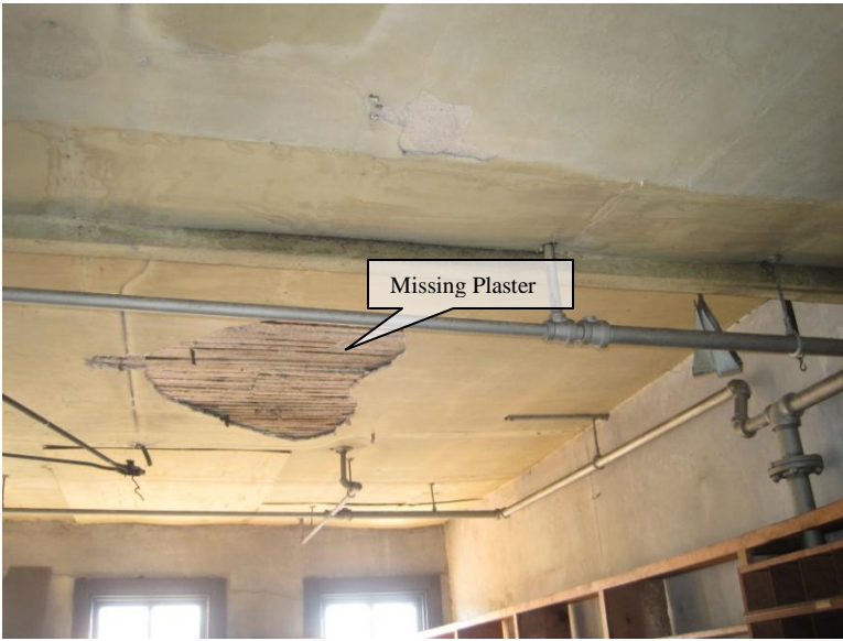
Figure 86. Third Floor: fallen plaster.
