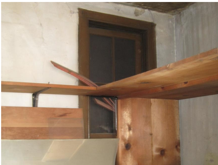
Figure 68. Third Floor: closed off north wall window.
