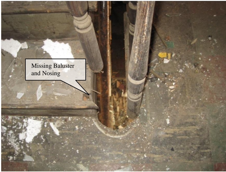
Figure 37. Second Floor: missing baluster and nosing.
