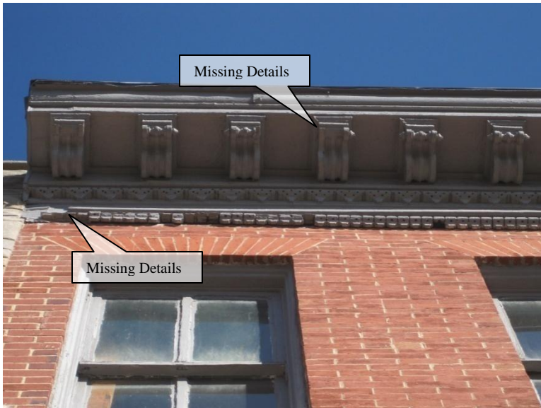
Figure 32. Exterior: missing details and cracking paint on cornice.
