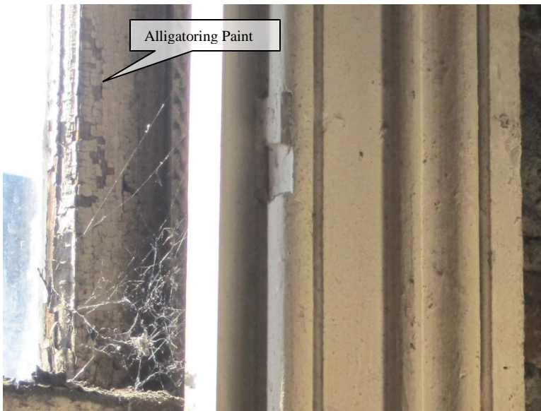
Figure 64. Second Floor: alligatoring paint on west window sash.
