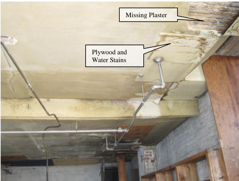
Figure 83. Third Floor: water damage and plywood patches on plaster ceiling.
