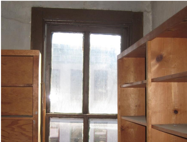
Figure 67. Third Floor: good condition of wood, paint, and glass on upper portions on west window.
