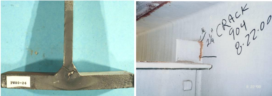
Figure 1.2 Typical Fatigue-induced Cracking
