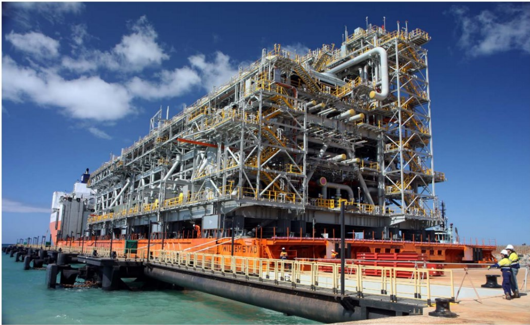
Figure 1.10: An acid gas removal unit (AGRU) module for the Gorgon LNG project on Barrow Island (Chevron Corporation, 2013).
