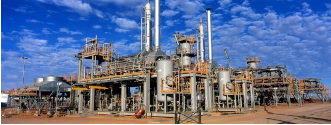
Figure 1.11: Amine-based CO 2 -separation system for natural gas sweetening at BP plant in In Salah, Algeria (In Salah Gas, 2014).
