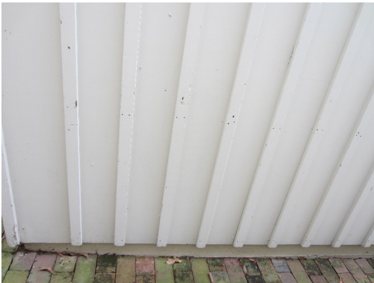
Figure 107: The detached battens on the southwest elevation.
