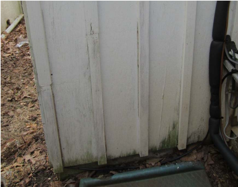
Figure 112: Worn paint with biological growth on the northwest elevation.
