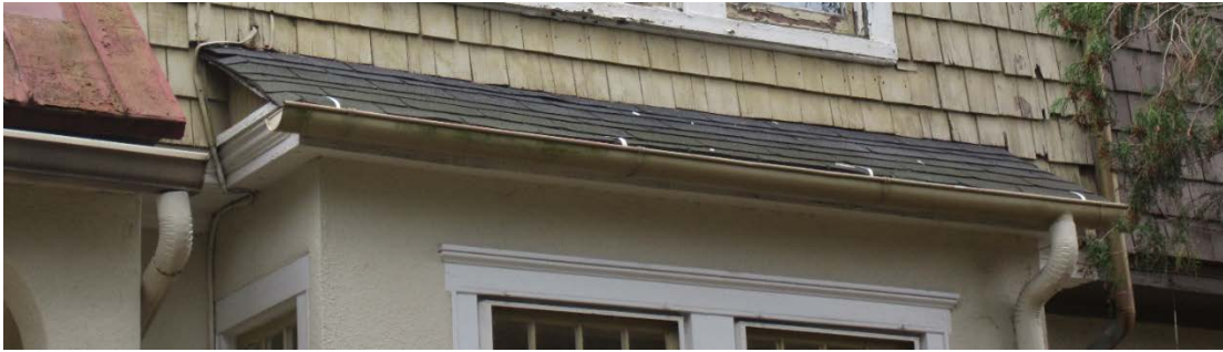
Figure 95: Biological growth on the low portion of the asphalt shingle roof on the square bay.
