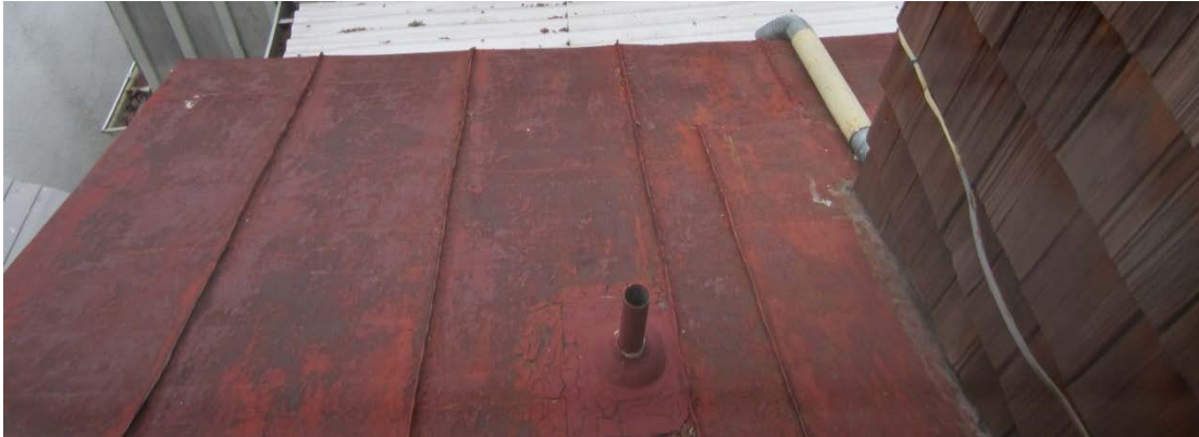
Figure 102: Part of the metal roof, showing the typical conditions of peeling paint and rust.
