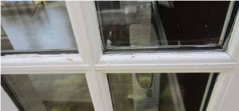
Figure 132: Minor peeling paint on one of the sidelights on the northwest elevation.
