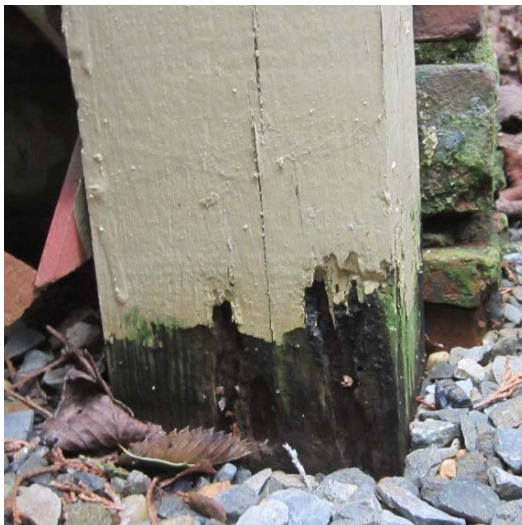
Figure 79: Deteriorating wood, peeling paint and biological growth on the western stair column.
