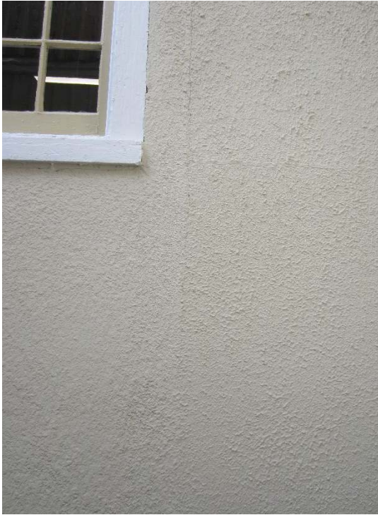
Figure 58: Vertical crack running from the second floor to the foundation on the southeast elevation.
