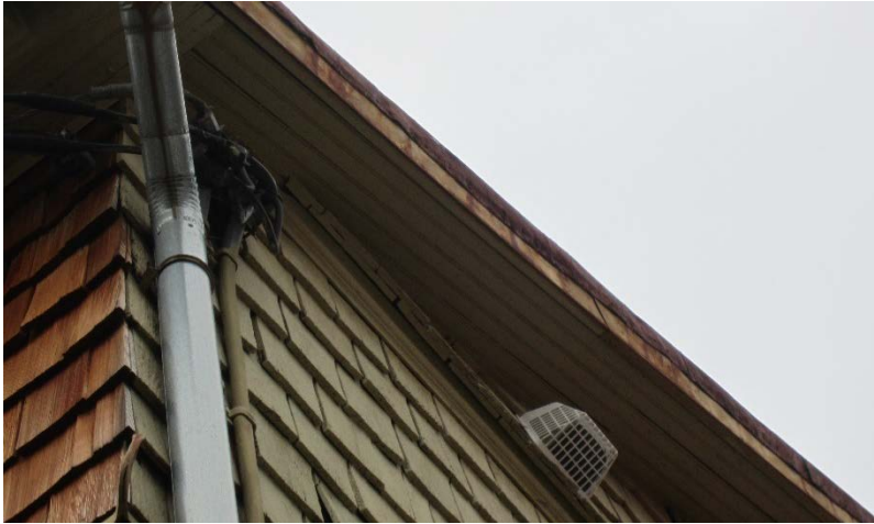
Figure 82: A detail of the rust staining on the fascia on the northeast elevation.
