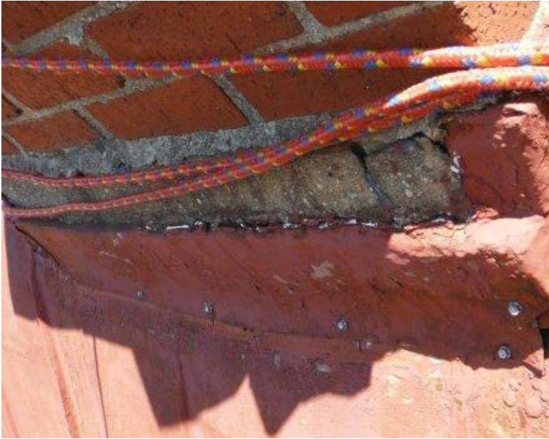
Figure 92: Missing metal flashing at the chimney. Photograph taken on June 8, 2013 and provided to the author by AIA Maryland.
