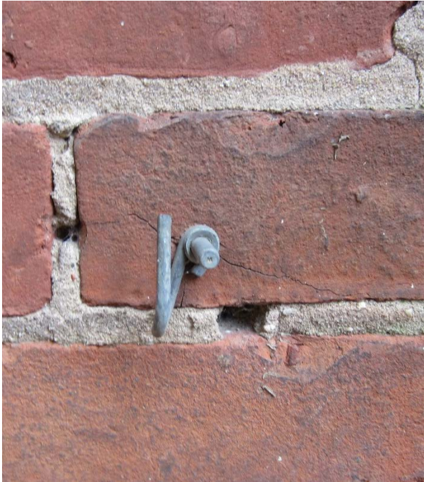
Figure 45: Metal anchor secured in brick with hairline crack radiating out from it.
