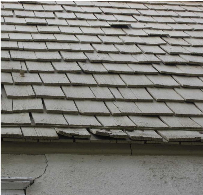
Figure 73: An example of some of the warped and raised shingles.
