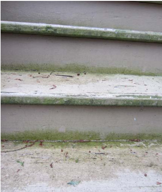
Figure 83: There is biological growth on the majority of the porch stairs.
