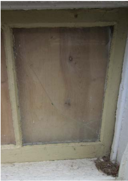
Figure 125: Broken glass pane in the basement window.
