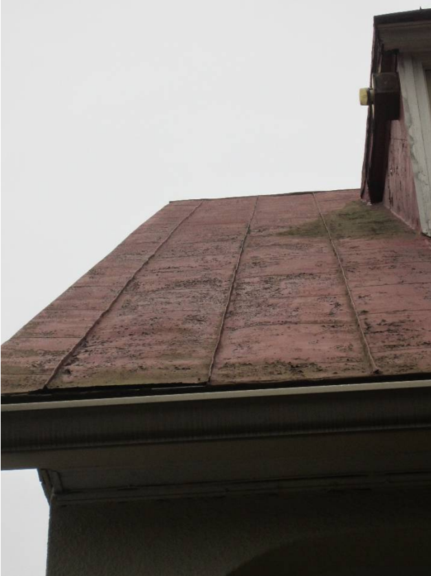
Figure 94: Biological growth on the roof.
