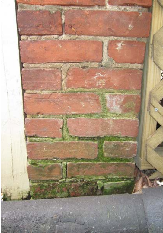
Figure 47: Biological growth on the bottom portion of the southwest elevation of the western brick porch pier.
