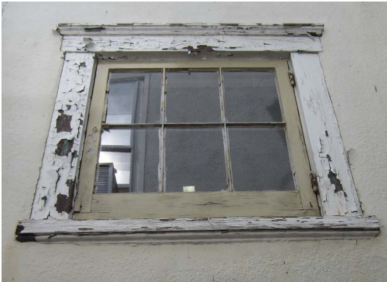
Figure 128: Northeast window on the small addition: with peeling paint and deteriorated glazing putty.
