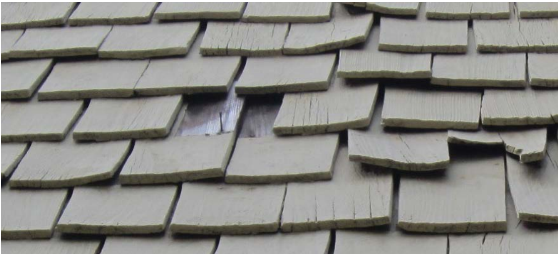
Figure 71: Missing shingles on the second floor on the northeast elevation.
