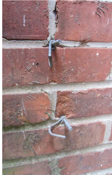
Figure 46: Metal anchors fastened in the mortar and the mortar cracking around it.
