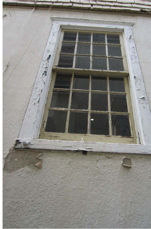
Figure 63: Peeling paint on the stucco below one of the windows on the northeast elevation.
