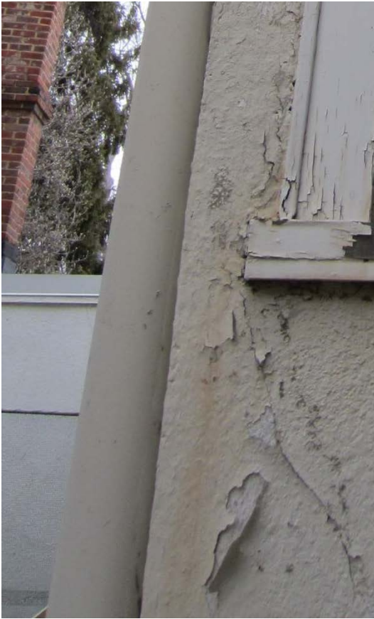
Figure 66: The water staining along the corner of the southwest elevation of the square bay and a close-up of the peeling paint.
