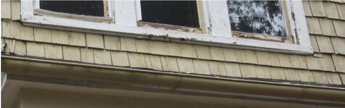
Figure 69: Minor deterioration in the shingles below the triple window on the northwest elevation.
