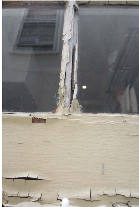
Figure 124: The eastern window on the first floor of the northeast elevation, which shows the typical condition of the glazing putty.
