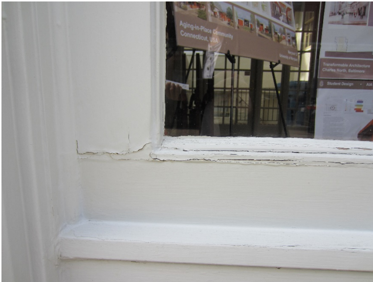
Figure 130: Hairline crack and peeling paint at the southern window.
