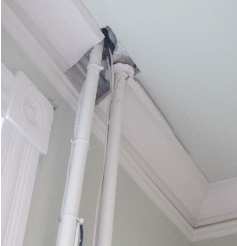
Figure 143: Detached crown molding in the southern corner.
