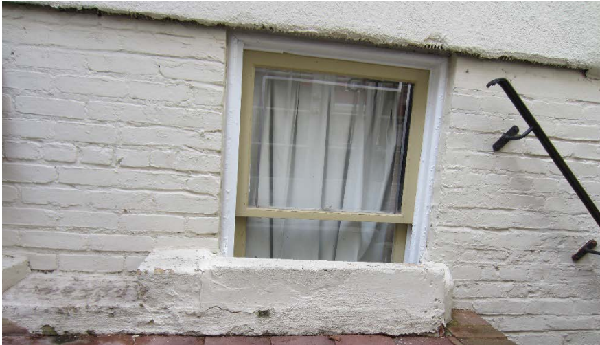
Figure 50: The only painted portion of the foundation.
