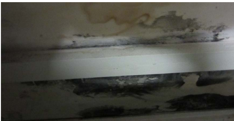
Figure 148: Mold and staining on the exterior wall of the closet.
