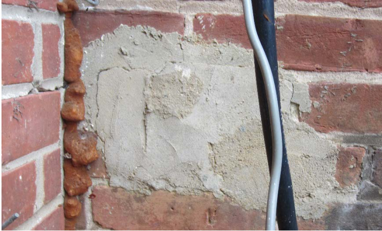
Figure 43: Mortar filling foundation hole and covering the surrounding bricks west of the square bay.
