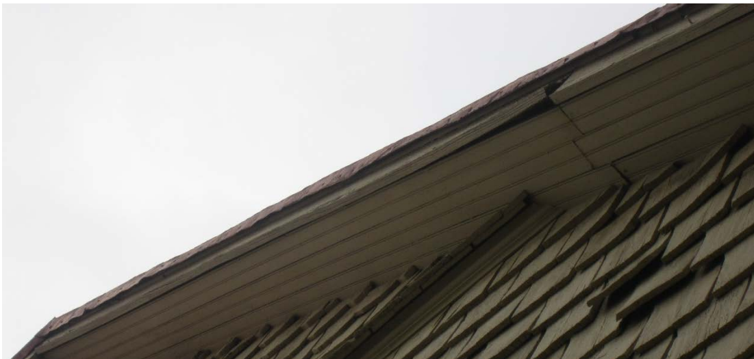
Figure 81: The portion of the fascia that is warped and loose on the northeast elevation.
