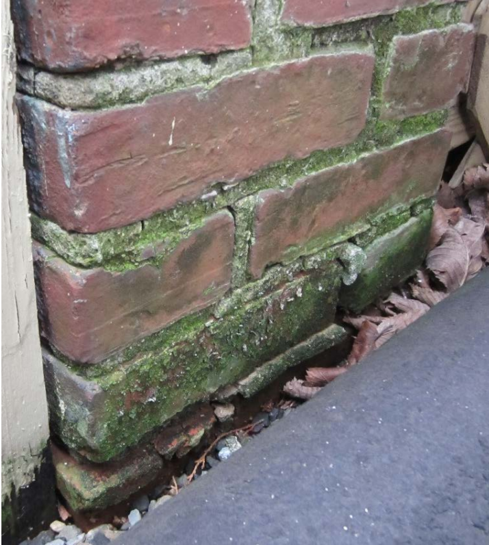
Figure 39: Cracking and deteriorated mortar on the bottom portion of the western brick porch pier on its southwest elevation.
