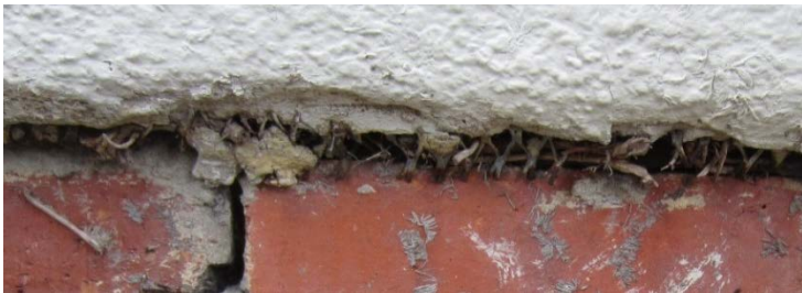
Figure 53: Exposed metal lath and deteriorating stucco west of the basement windows on the square bay.
