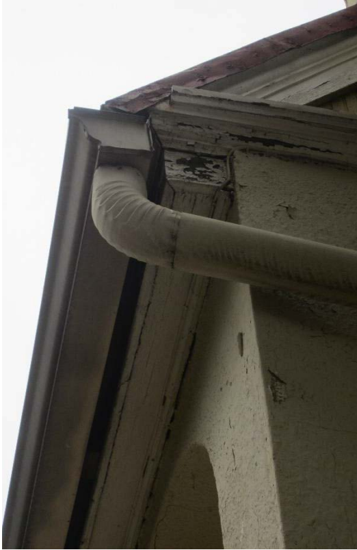
Figure 77: The deteriorating wood and peeling paint on the porch soffit on the northwest elevation and the trim on the southwest.
