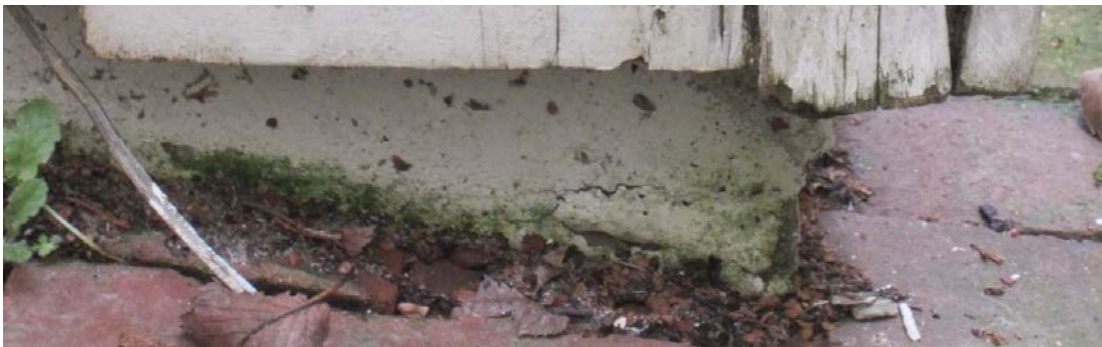
Figure 103: Biological growth on the concrete slab-on-grade.
