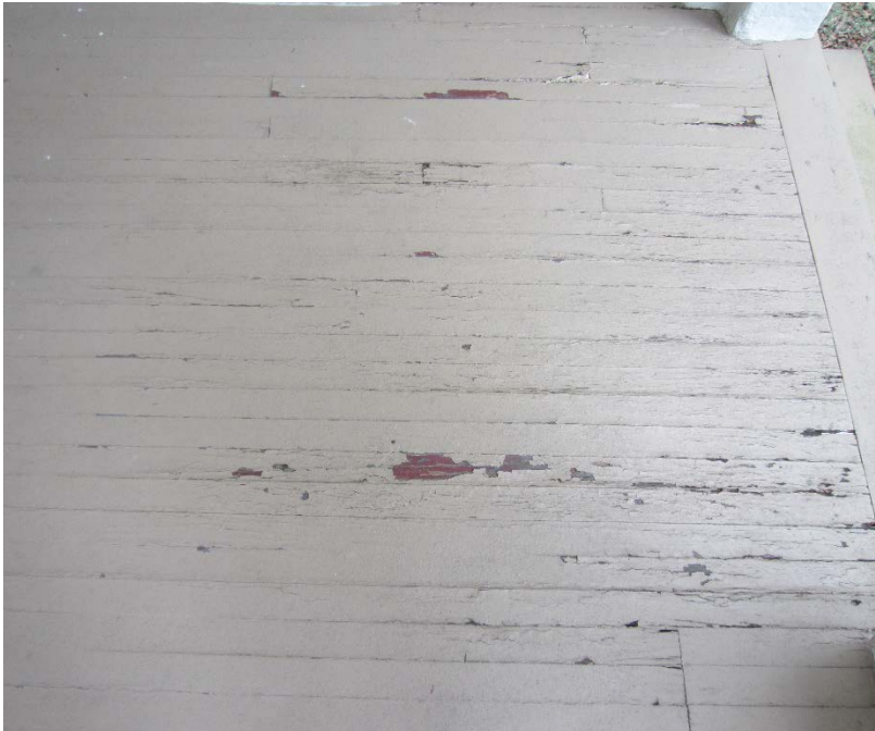
Figure 76: Deteriorated boards and peeling paint on the porch floor.
