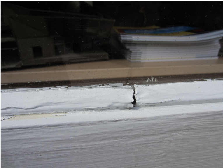
Figure 135: Crack in glazing putty.
