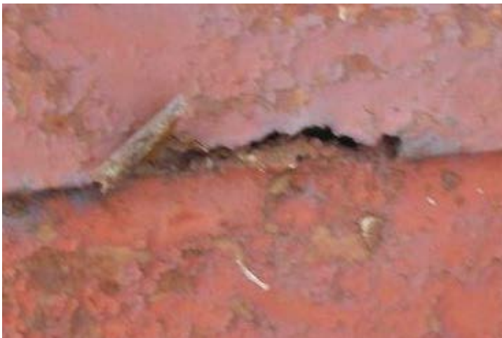
Figure 88: Example of a broken seam. Photograph taken on June 8, 2013 and provided to the author by AIA Maryland.
