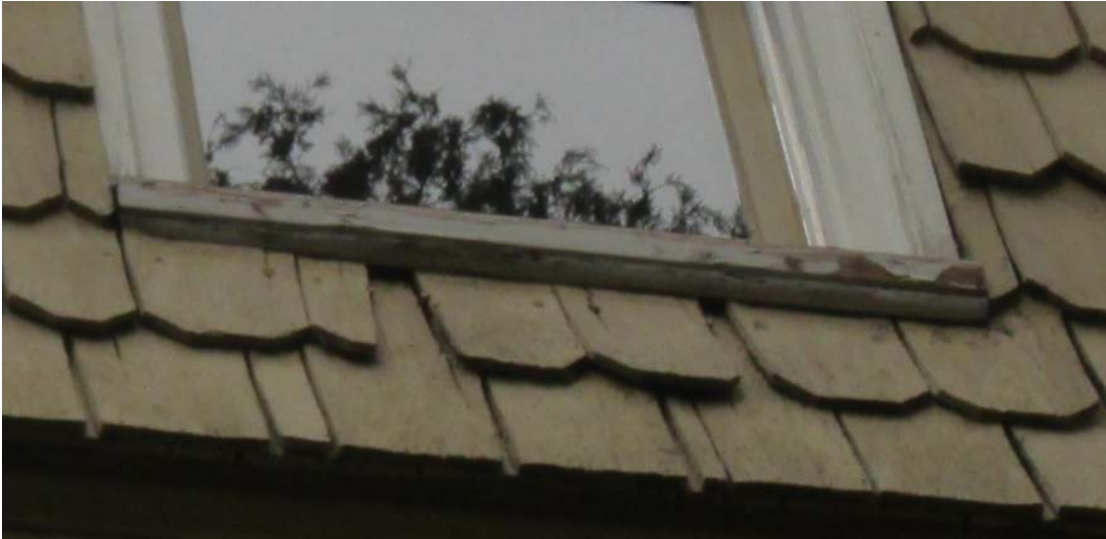
Figure 70: Partially missing shingles under the third floor / attic window in cross gable on the northwest elevation.
