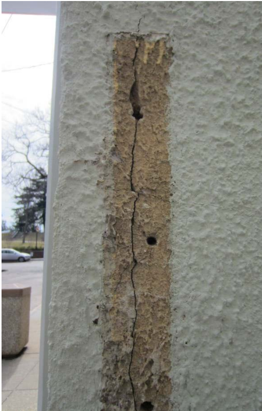
Figure 104: A portion of the damage to the stucco caused by a piece of wood that was formerly attached to the northeast elevation.
