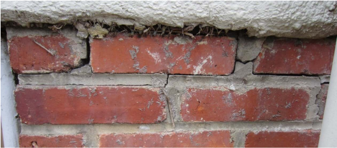
Figure 35: Cracking mortar west of the basement windows on the square bay; episodes of improper repointing are also evident.
