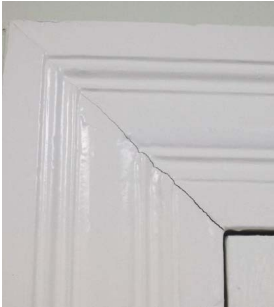
Figure 151: The historic door trim in the conference rooms serves as an example of a crack in a mitered joint.
