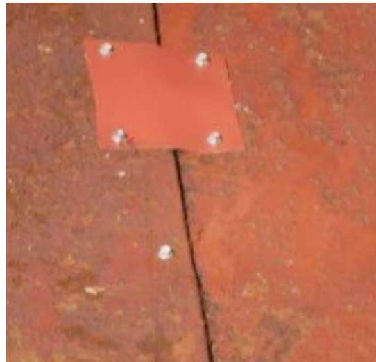
Figure 91: Examples of an improper roof repair at a seam. Photograph taken on June 8, 2013 and provided to the author by AIA Maryland.
