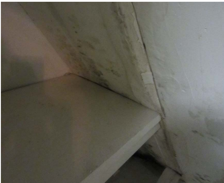
Figure 147: A portion of the mold on the exterior wall.
