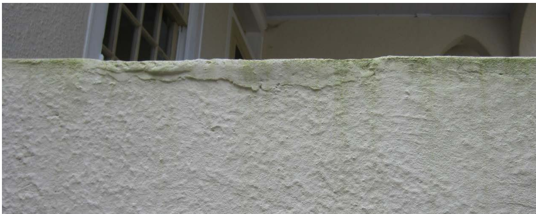
Figure 67: Biological growth along the porch railing.
