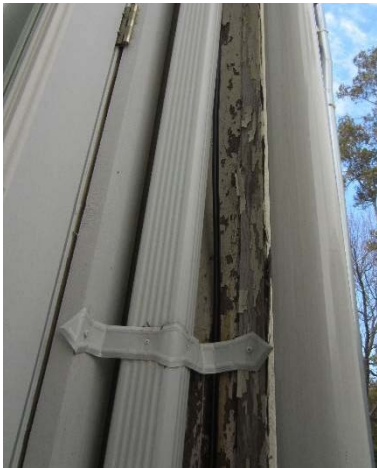
Figure 100: A portion of the peeling paint and deteriorated wood at the corner between the small and commercial additions.
