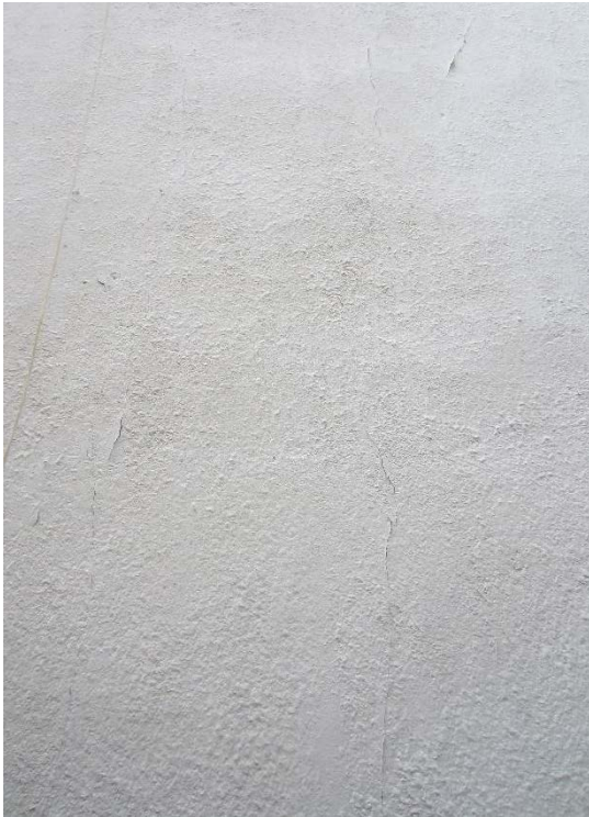
Figure 56: Vertical cracks north of the northeast elevation first floor windows. The cracks run from the foundation to the second floor.
