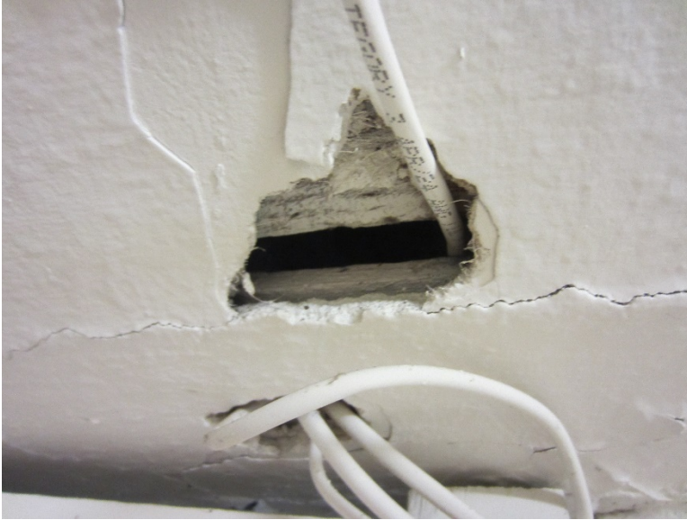
Figure 137: Two of the holes and radiating cracks in the basements plaster ceiling; both made to run wiring.
