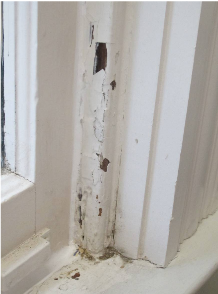
Figure 142: A close-up of the peeling paint on the window trim.
