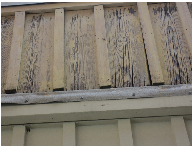
Figure 109: Deteriorated boards above the courtyard door on the northwest elevation.
