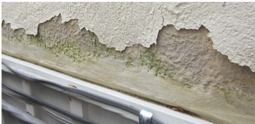
Figure 99: Peeling paint, exposed brown coat, and biological growth on the northeast elevation.
