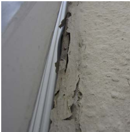
Figure 97: The typical condition of the peeling paint along the corner between the small and commercial additions.
