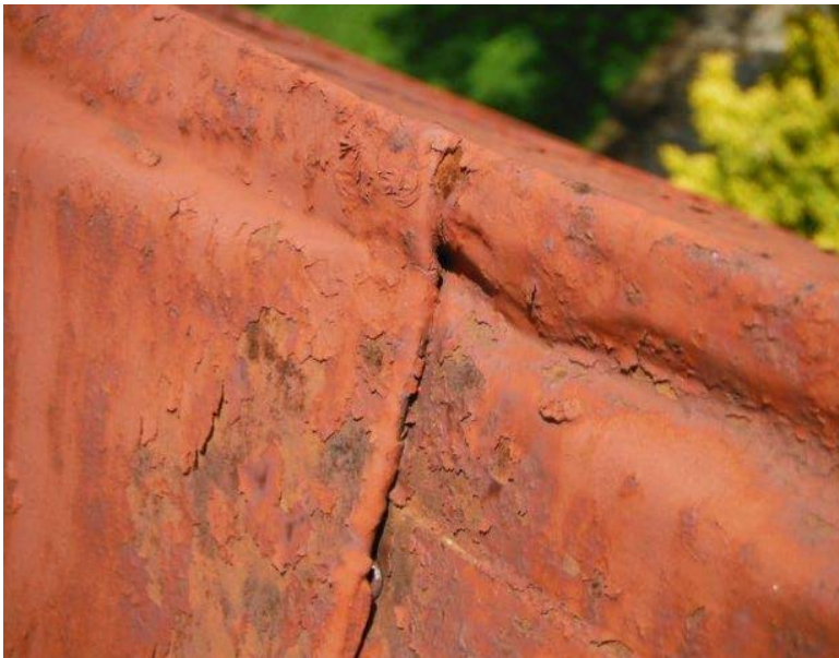
Figure 85: A close-up example of the peeling paint throughout the entire roof. Photograph taken on June 8, 2013 and provided to the author by AIA Maryland.
