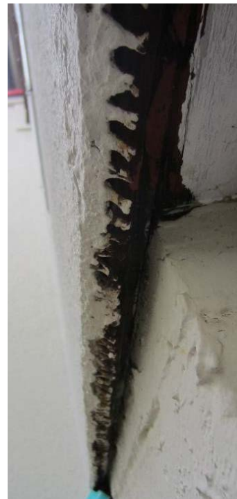
Figure 55: Exposed metal lath along the bottom of the stucco on the southeast façade.
