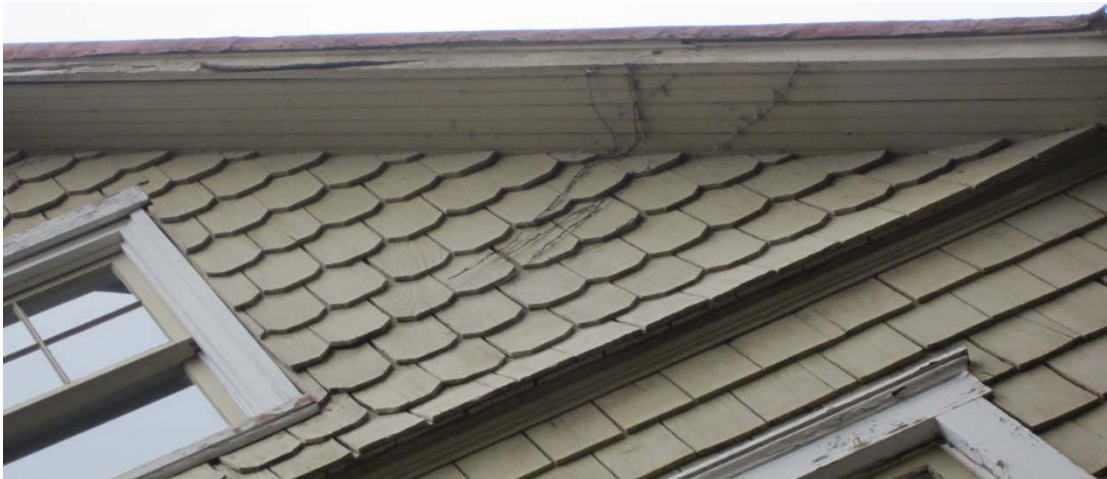
Figure 75: A close-up of one of the locations with dead organic matter.
