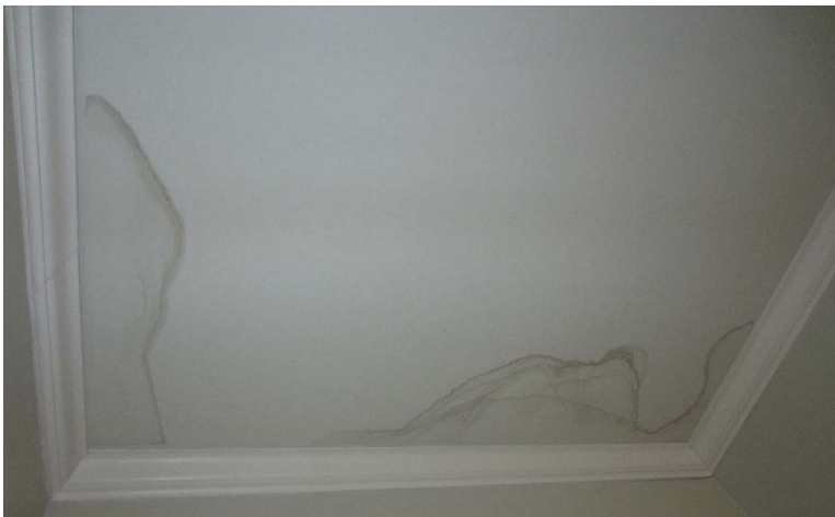
Figure 144: Water stains in the ceiling along the exterior wall.
