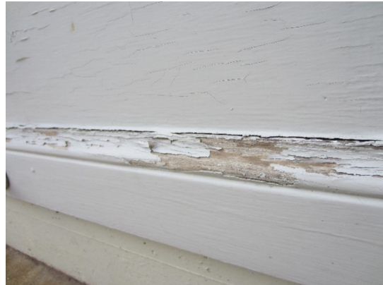
Figure 114: The peeling paint on the lower trim of the southern panel.
