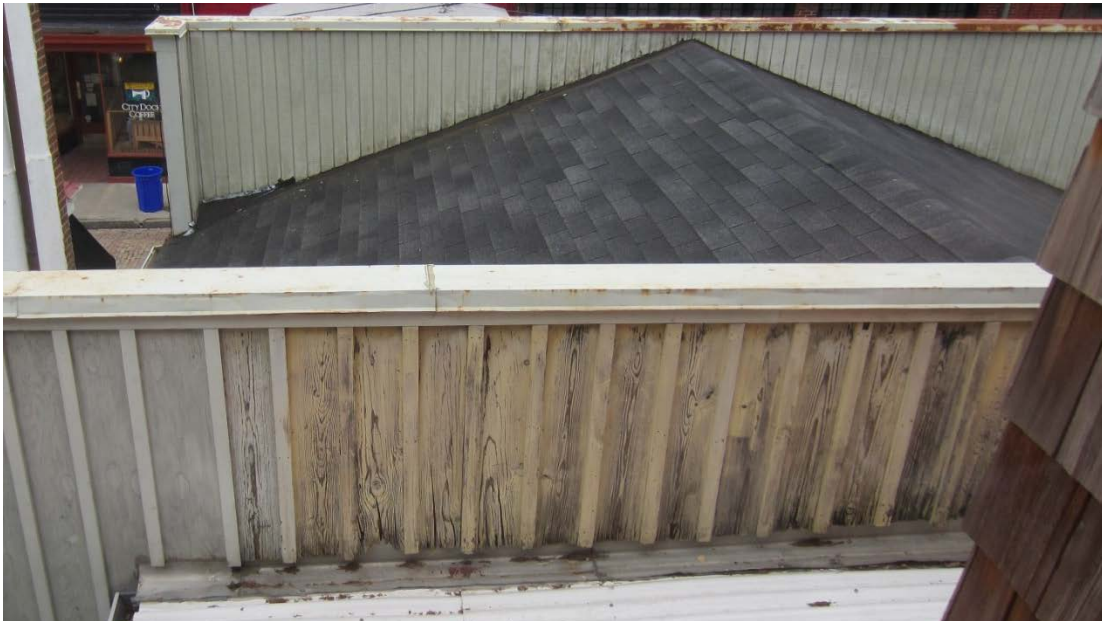
Figure 117: The current condition of the corrugated fiberglass and asphalt roofs with the rusted parapet caps.
