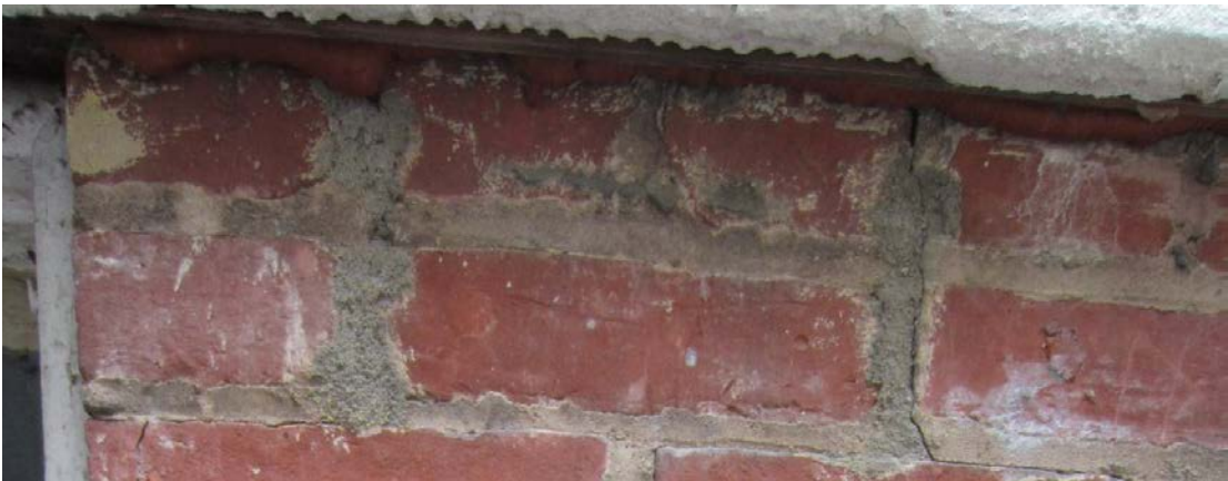
Figure 36: Repointing that tried to repair some cracks, but did not fix them on the northwest elevation, north of the basement window.
