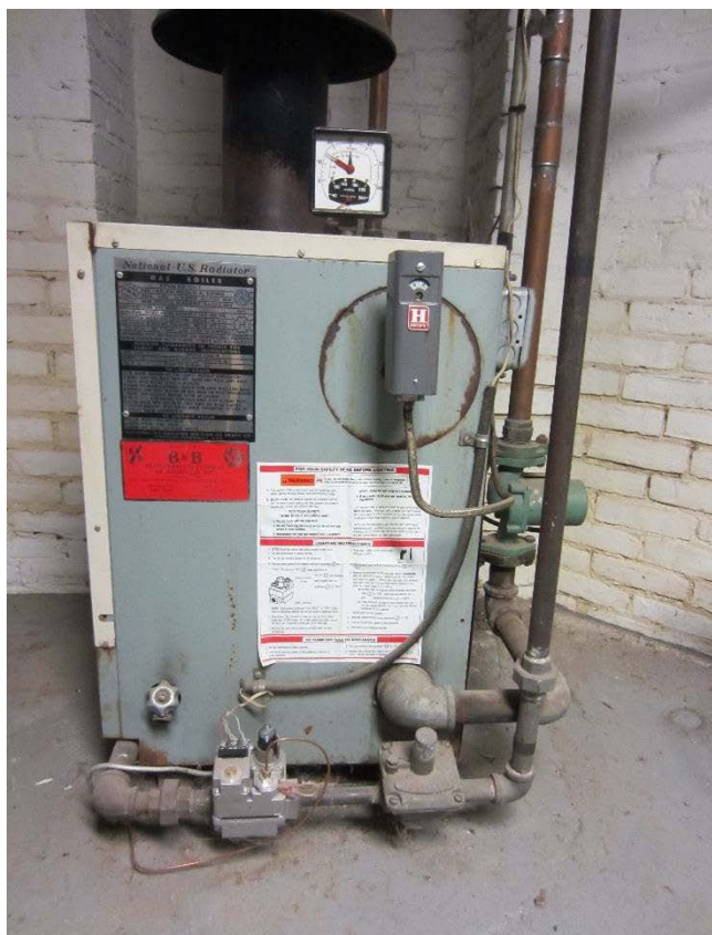
Figure 23: Old gas boiler by the National-US Radiator Division of Crane Company still installed in the basement.
