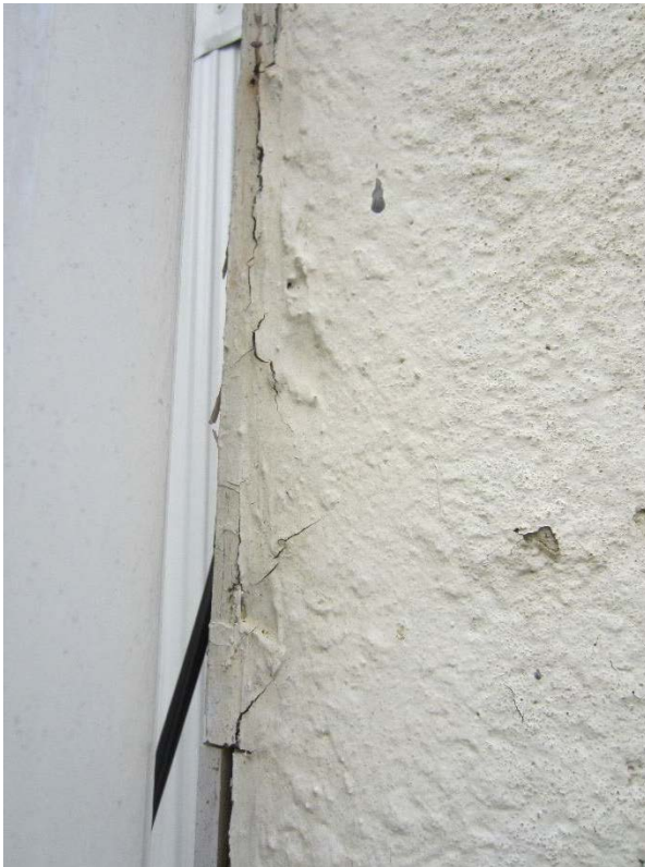
Figure 96: A close-up of the crack that is along the full length of the corner between the small and commercial additions.
