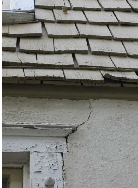
Figure 59: Example of the stress cracks at the two first floor windows on the northeast elevation.
