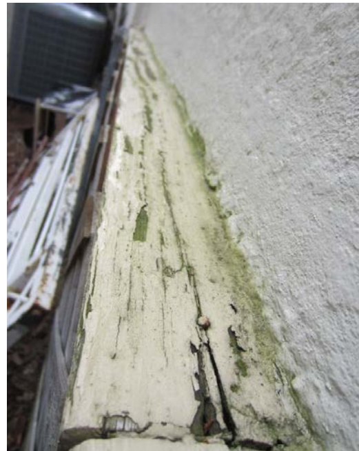
Figure 84: Biological growth is evident on the wood along the edge of the stucco on the northeast elevation of the porch. This image also shows the extent of the deterioration and peeling paint on this element.
