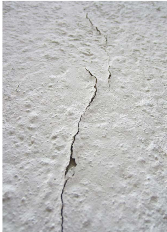
Figure 57: Close-up of the vertical cracks on the northeast elevation.
