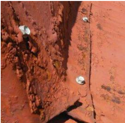
Figure 90: Roof repair in the flashing at the chimney. Example of improper repair with stainless steel screws. Photograph taken on June 8, 2013 and provided to the author by AIA Maryland.
