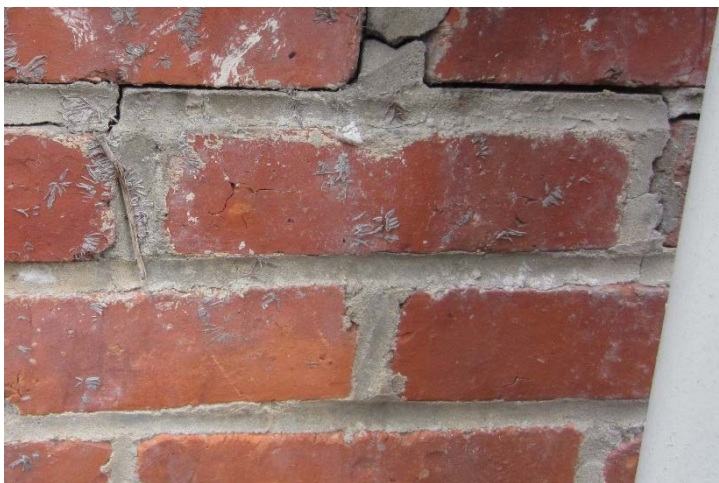
Figure 40: Evidence of poor repointing on the square bay west of the basement windows. The mortar is covering the bricks.
