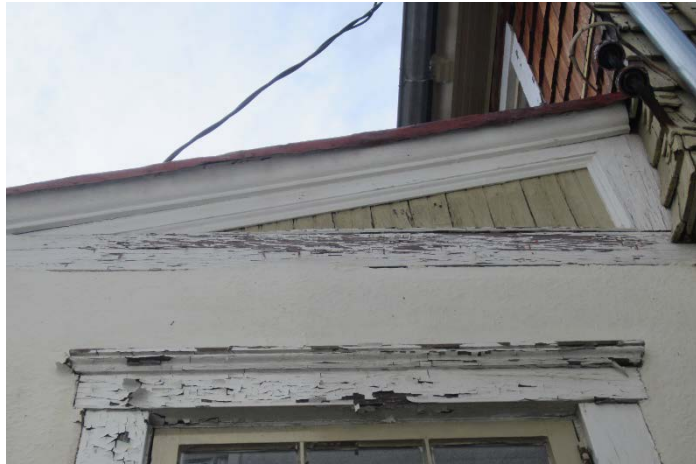
Figure 101: The peeling paint and deteriorated wood above the stucco on the northeast elevation.
