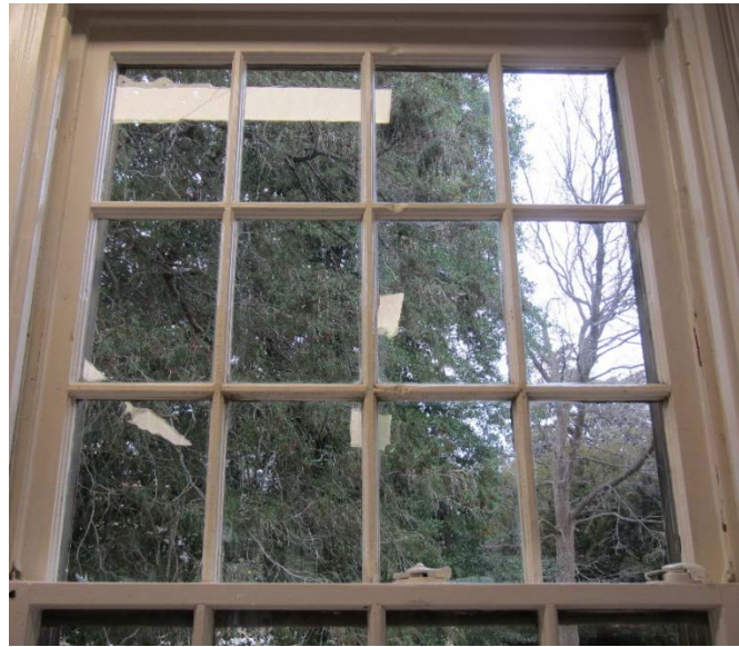
Figure 126: The three broken panes of glass are in the corners of the top sashes excluding one on the upper right.
