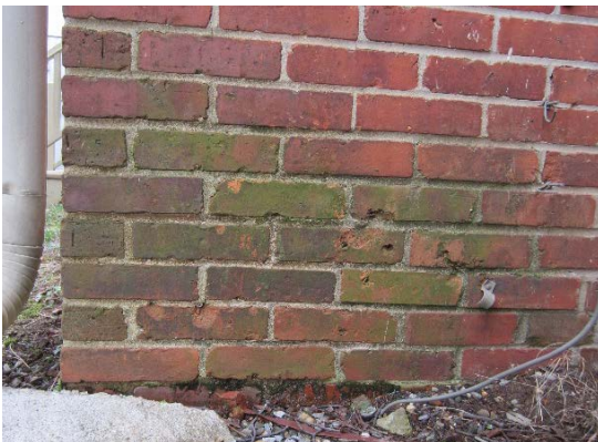
Figure 49: Biological growth on a portion of the southwest elevation of the square bay.
