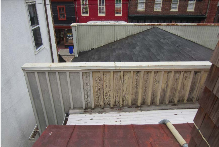
Figure 110 Primed but unpainted parapet on the northwest elevation.
