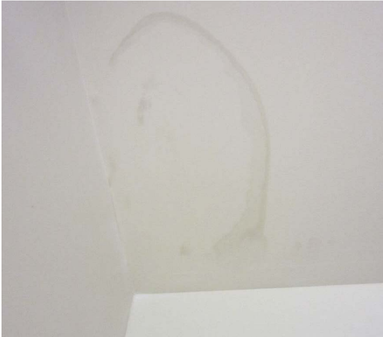
Figure 149: Water staining on the wall above closet door.
