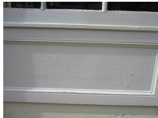
Figure 116: Peeling paint on the northern panel.
