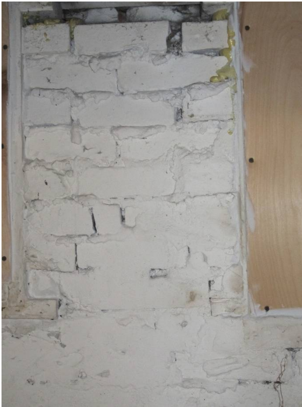
Figure 136: Deteriorated mortar in the basement.
