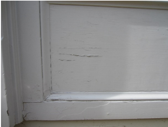
Figure 113: Typical condition of the peeling paint in the recessed panels.
