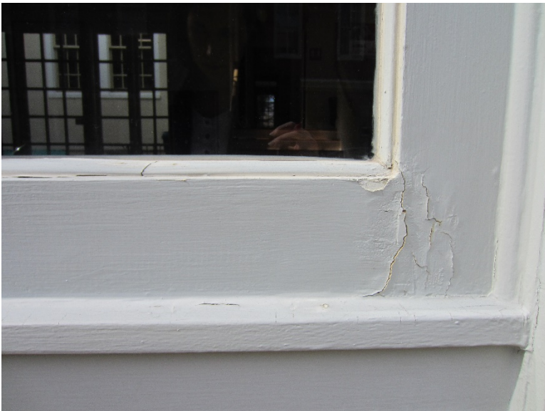
Figure 133: Peeling paint on the southern window sash.
