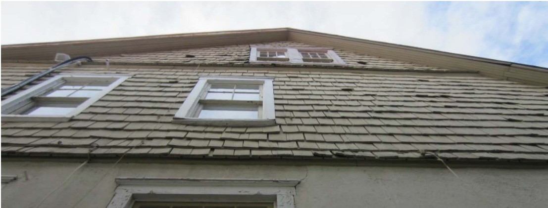
Figure 72: The warped and raised shingles on the northeast elevation.
