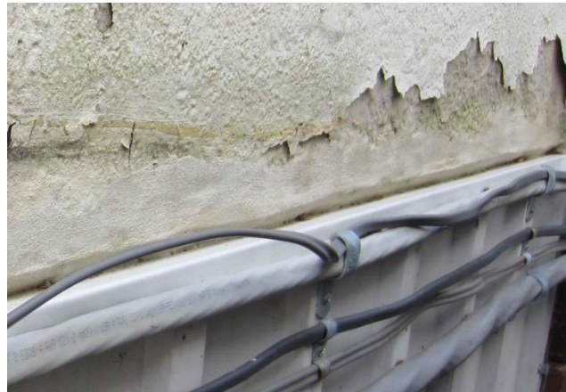
Figure 98: An example of the peeling paint, exposed brown coat, and biological growth on the bottom of the northeast elevation.
