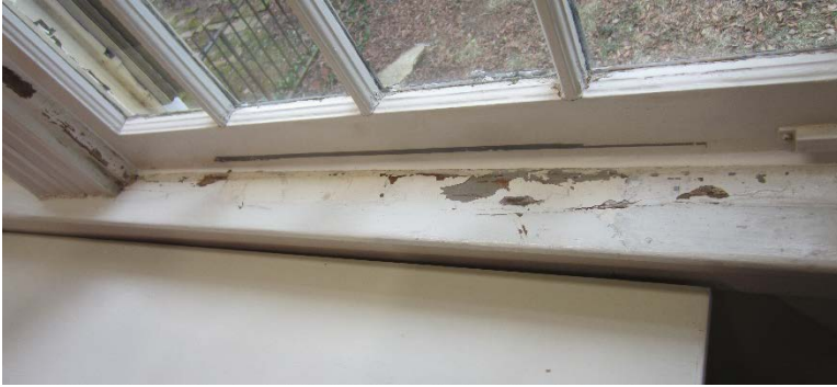
Figure 141: The peeling paint on the window sill on the northern window.
