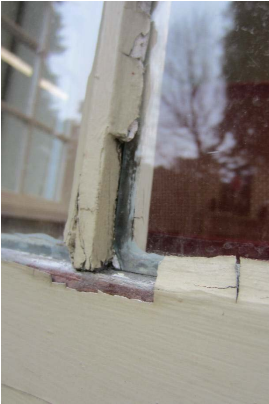
Figure 123: Northern first floor window on the square bay which is an examples of the deterioration of the glazing putty.
