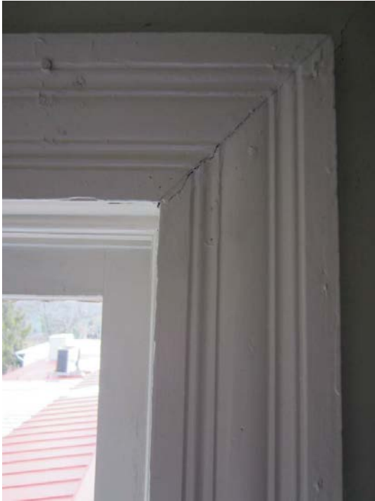
Figure 154: Historic window trim in the northeastern room is an example of a crack in mitered joint.
