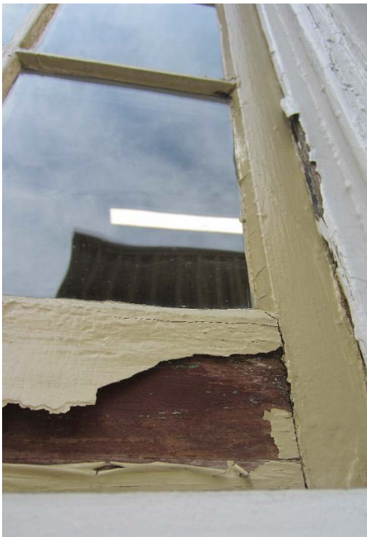
Figure 121: The southern window on the first floor of the southeast is an example of the typical peeling paint found on the window sashes.
