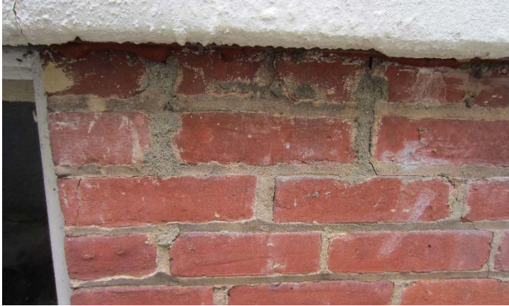
Figure 41: Improper repointing on the northeast foundation to the north of the basement window. The mortar is a different color and the joint is too wide.
