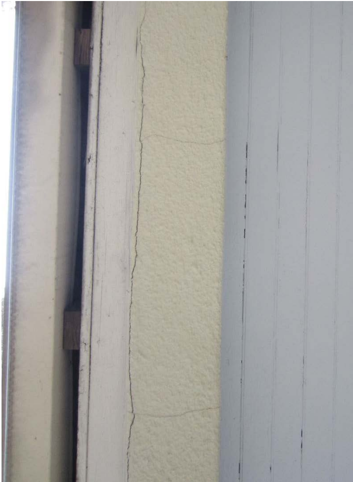
Figure 61: Crack along the edge of the flat portion of the porch opening.
