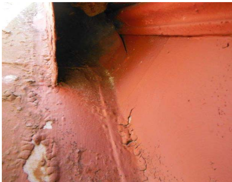
Figure 86: Example of the blistered and peeling paint on the roof. Photograph taken on June 8, 2013 and provided to the author by AIA Maryland.
