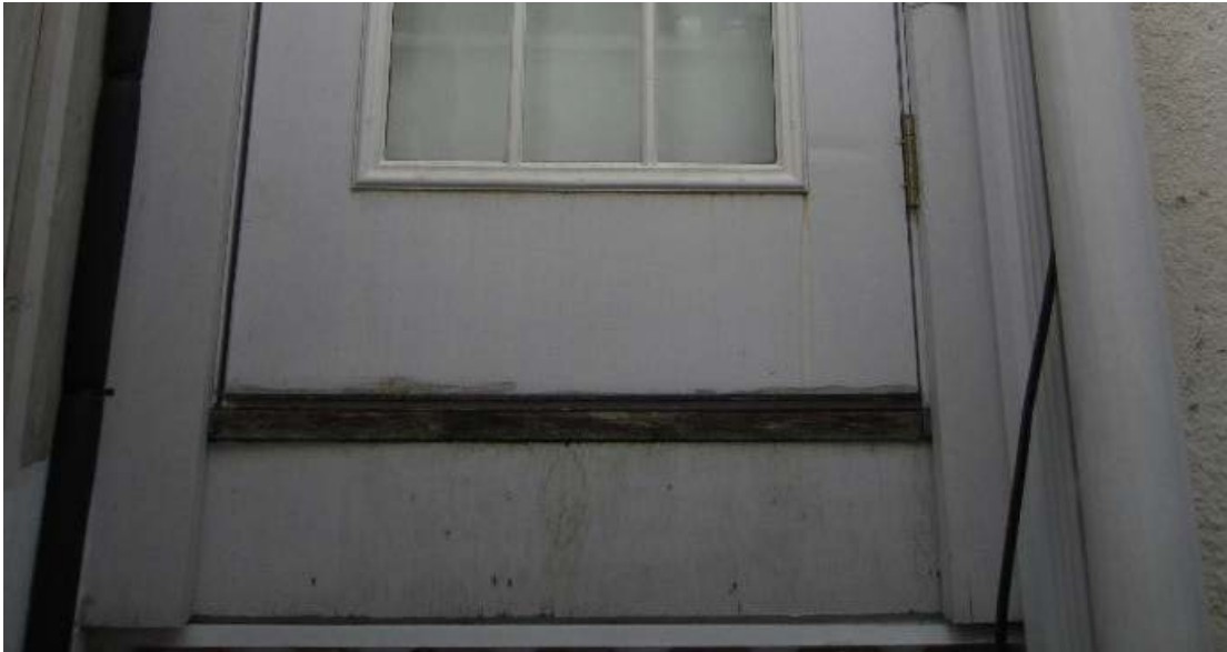
Figure 129: Deteriorated sill and rust staining on the fixed door.
