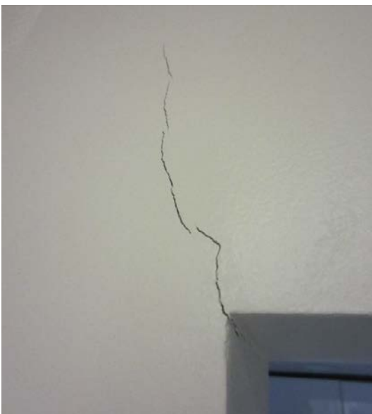
Figure 153: Stress crack at the opening between the transverse hall and kitchenette.
