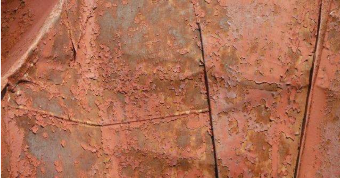
Figure 87: An example of the typical condition of the standing seam metal roof, showing the peeling paint and corrosion of the metal. Photograph taken on June 8, 2013 and provided to the author by AIA Maryland.
