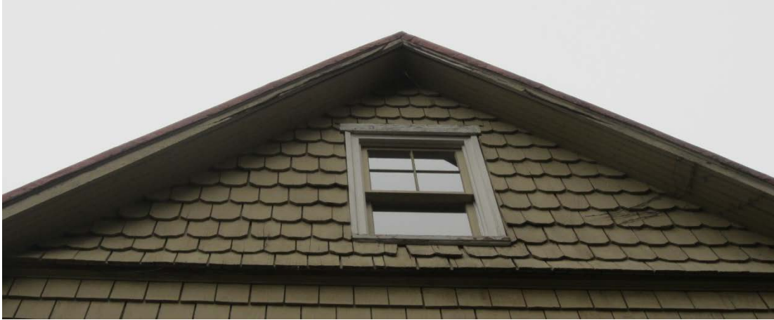
Figure 80: The wood for the fascia is deteriorating on both sides at the cross gable.
