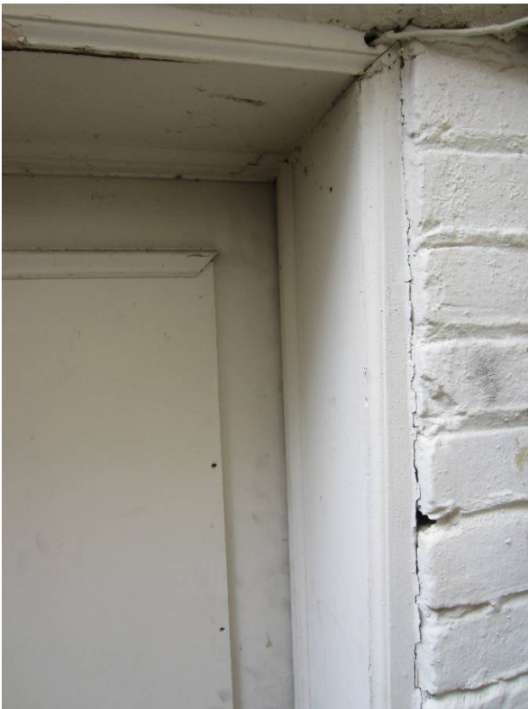
Figure 118: Close-up of the crack between the door and the foundation, and the opening in the header.
