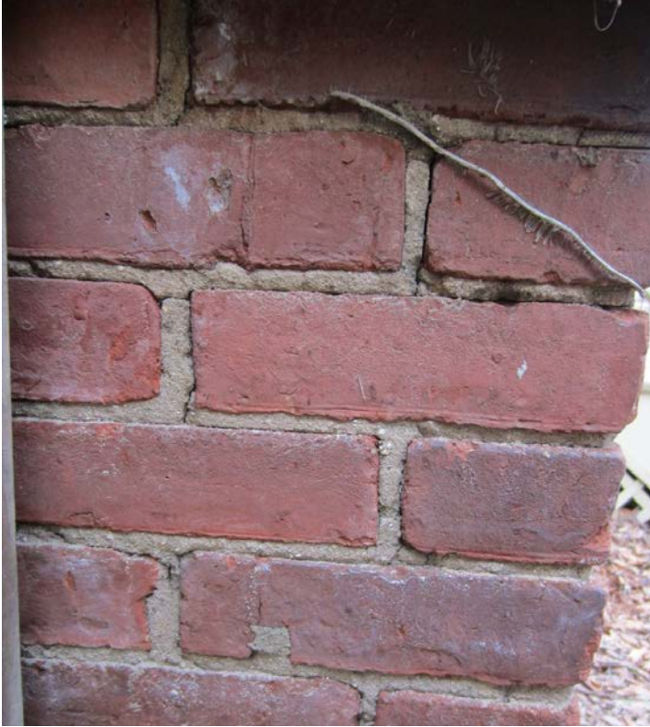
Figure 37: Cracking and deteriorated mortar on the northern brick porch pier, northeast elevation. In addition, dead organic matter is still attached to the brick.
