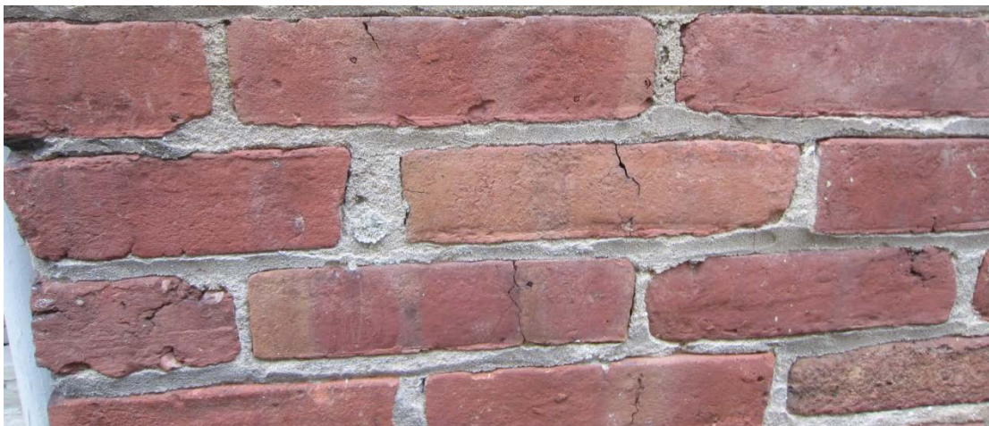
Figure 34: Bricks cracking north of the basement window on northwest elevation.
