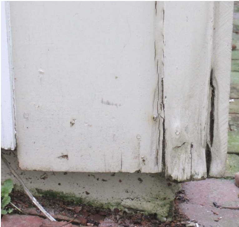
Figure 108: Deteriorated wood and peeling paint on the eastern corner.
