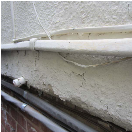
Figure 64: A portion of the peeling paint along the bottom of the northeast elevation.
