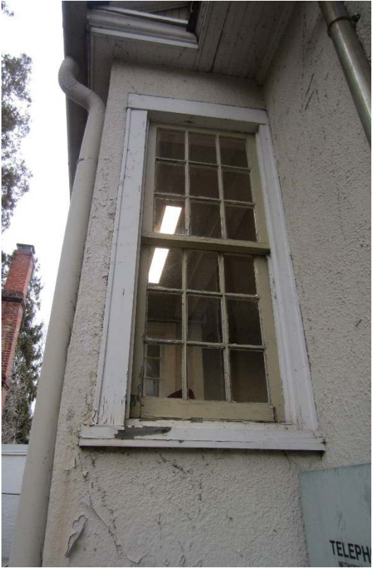
Figure 62: Peeling paint below the window on the southwest elevation of the square bay.
