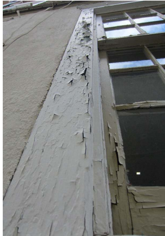
Figure 120: Northern window on the first floor of the northwest elevation, showing the typical condition of peeling paint on the windows.
