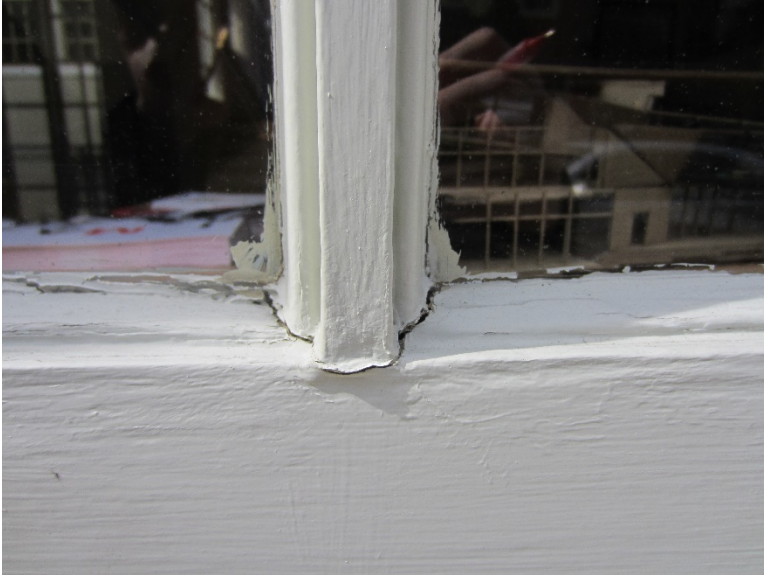
Figure 134: Crack in the glazing putty and around the muntin.
