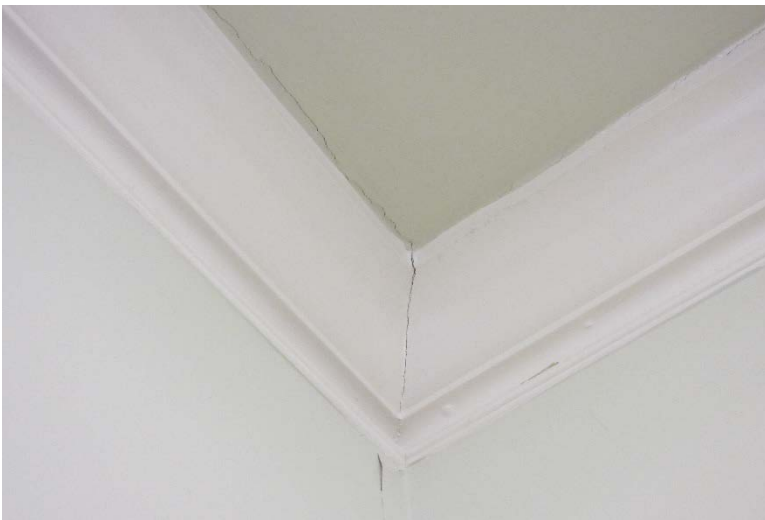
Figure 150: Crack running along the ceiling and through the crown molding in the eastern corner.
