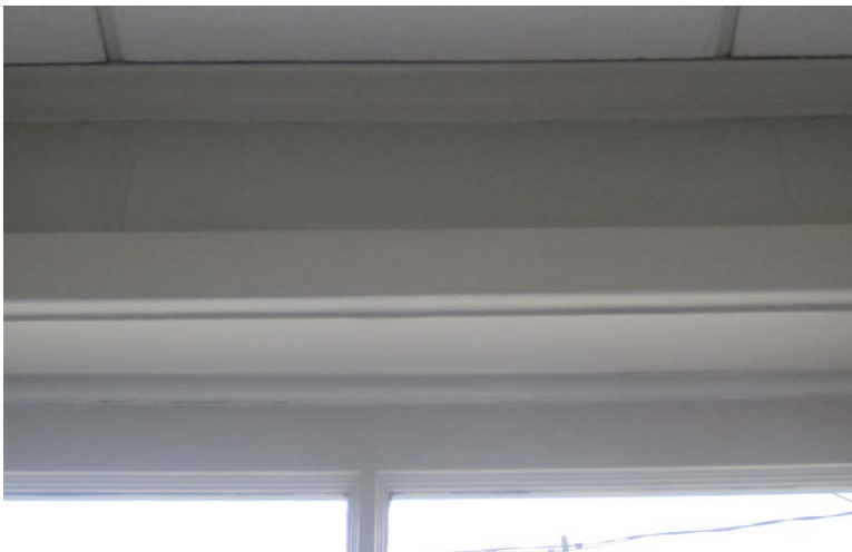
Figure 146: Two cracks above the northern window.
