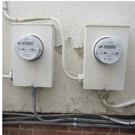
Figure 65: The peeling paint under the electrical meters on the northeast elevation. In addition, the northern meter has pulled away from the wall.
