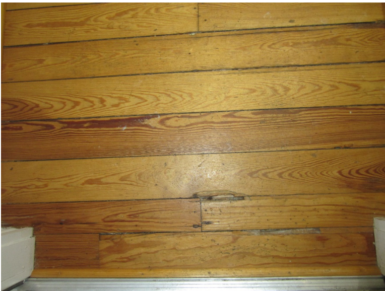
Figure 140: Deteriorated floorboards near the door separating the hall in the eastern set of the rooms.
