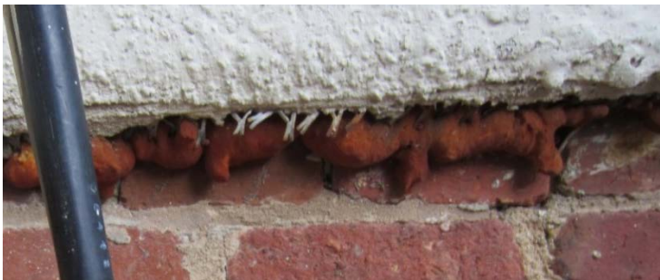
Figure 54: Exposed metal lath west of the square bay.
