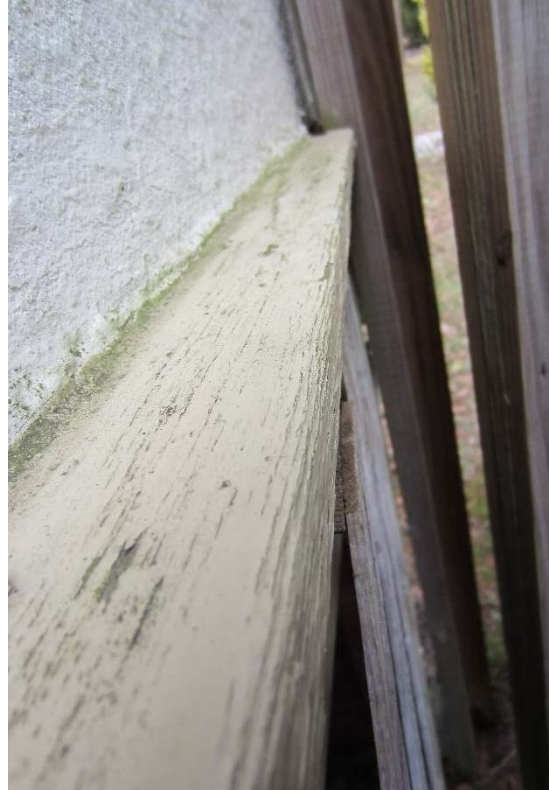
Figure 78: Deteriorating wood and peeling paint on the trim where the stucco is terminated on the northeast elevation of the porch.
