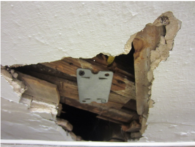
Figure 138: The worst of the holes in the basement plaster ceiling.
