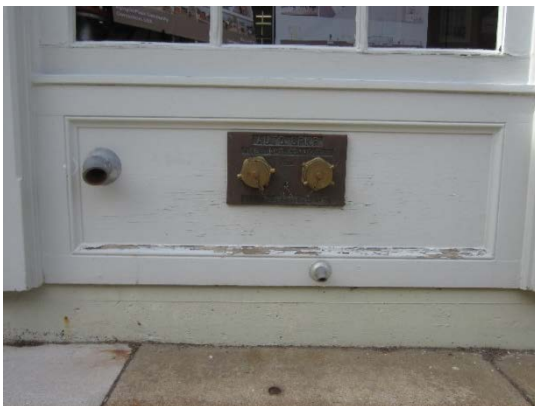
Figure 115: The peeling paint throughout the southern panel.
