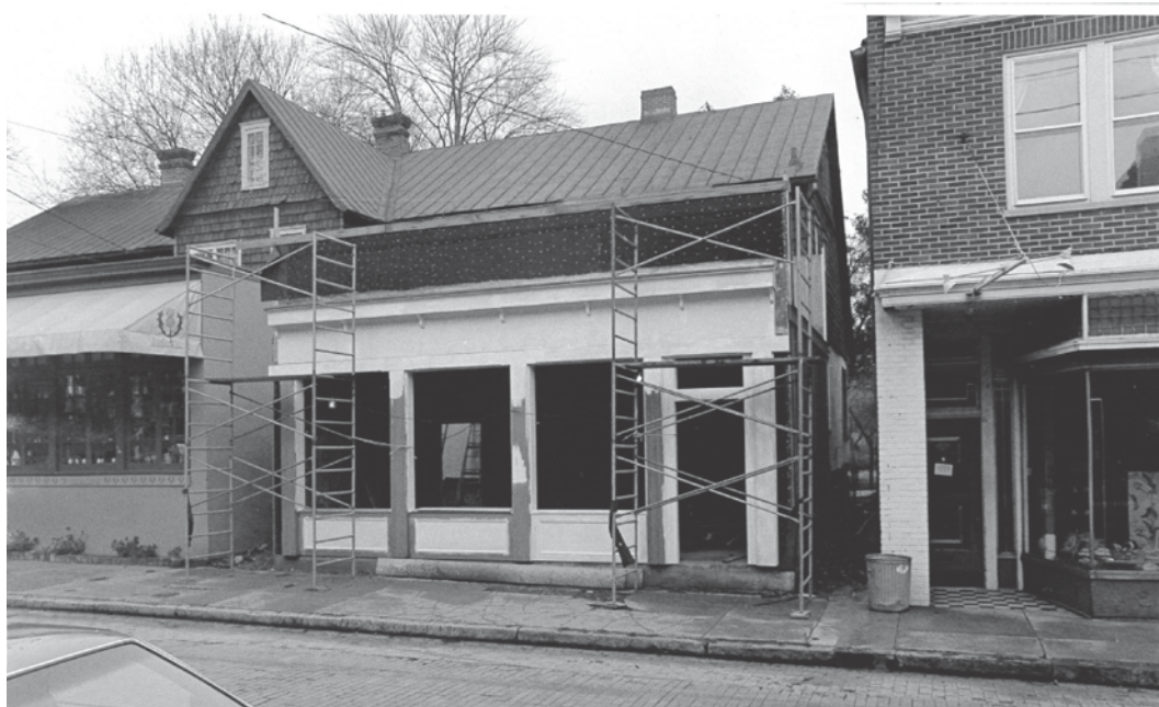
Figure 8: 1980 photograph of 86 Maryland Avenue's commercial addition under construction (Historic Annapolis Foundation Archives).
