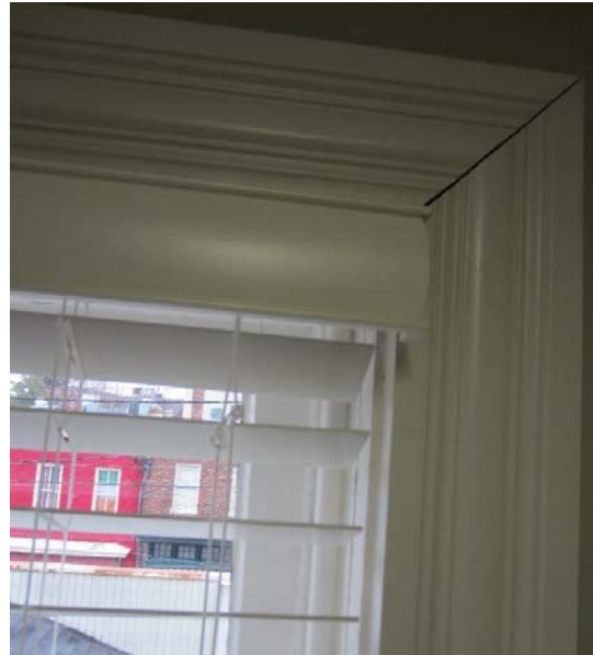
Figure 152: The new window trim in the southern office is an example of separation in a mitered joint.
