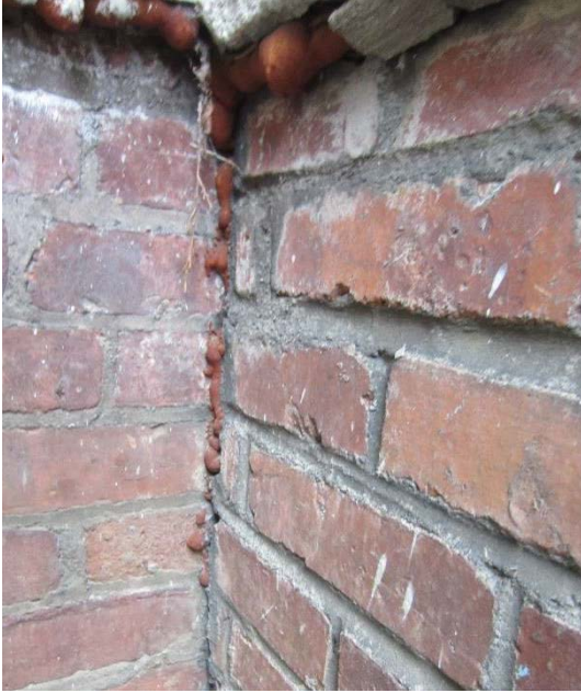
Figure 32: Northern corner where the square bay foundation connects with the main foundation. Spray foam insulation fills the openings caused by the settling.
