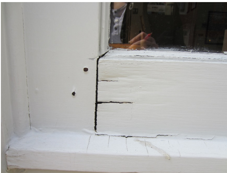
Figure 131: Separation at the sash joint at the center window.
