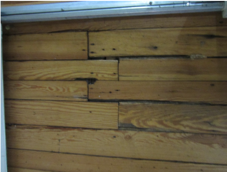
Figure 139: Deteriorated floorboards in the stair hall.
