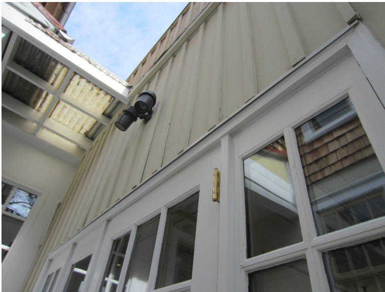
Figure 106: The seven detached battens on the northwest elevation.
