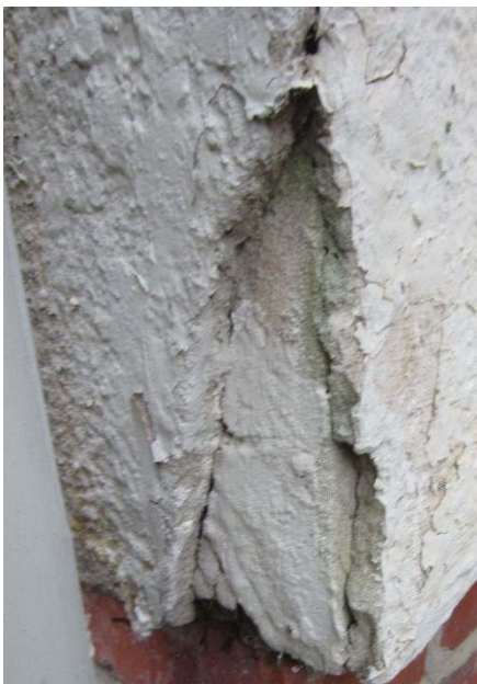
Figure 60: Missing outer coats of stucco exposing the scratch coat.
