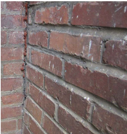
Figure 51: Paint splatter on the northeast face of the square bay.
