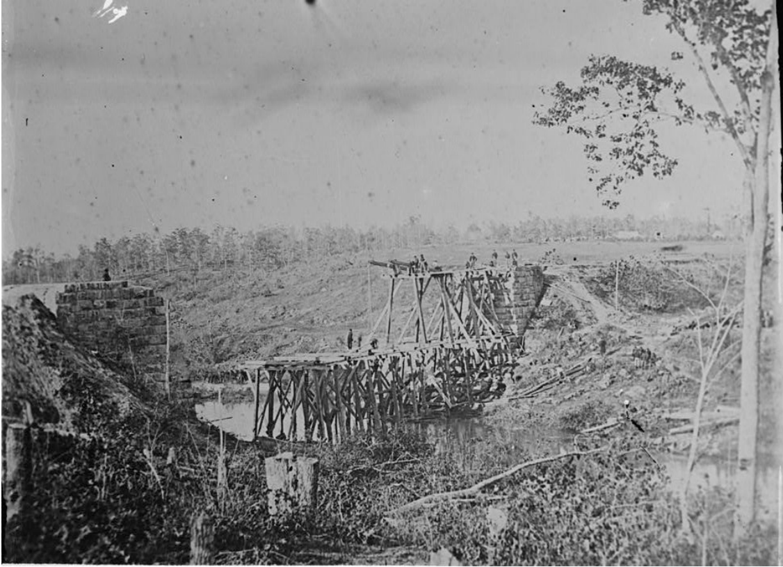
Figure 12: "Catlett's Station, Va., vicinity. Federal soldiers rebuilding the Orange & Alexandria Railroad bridge over Cedar Run," 1863 (Library of Congress Prints and Photographs Division).
