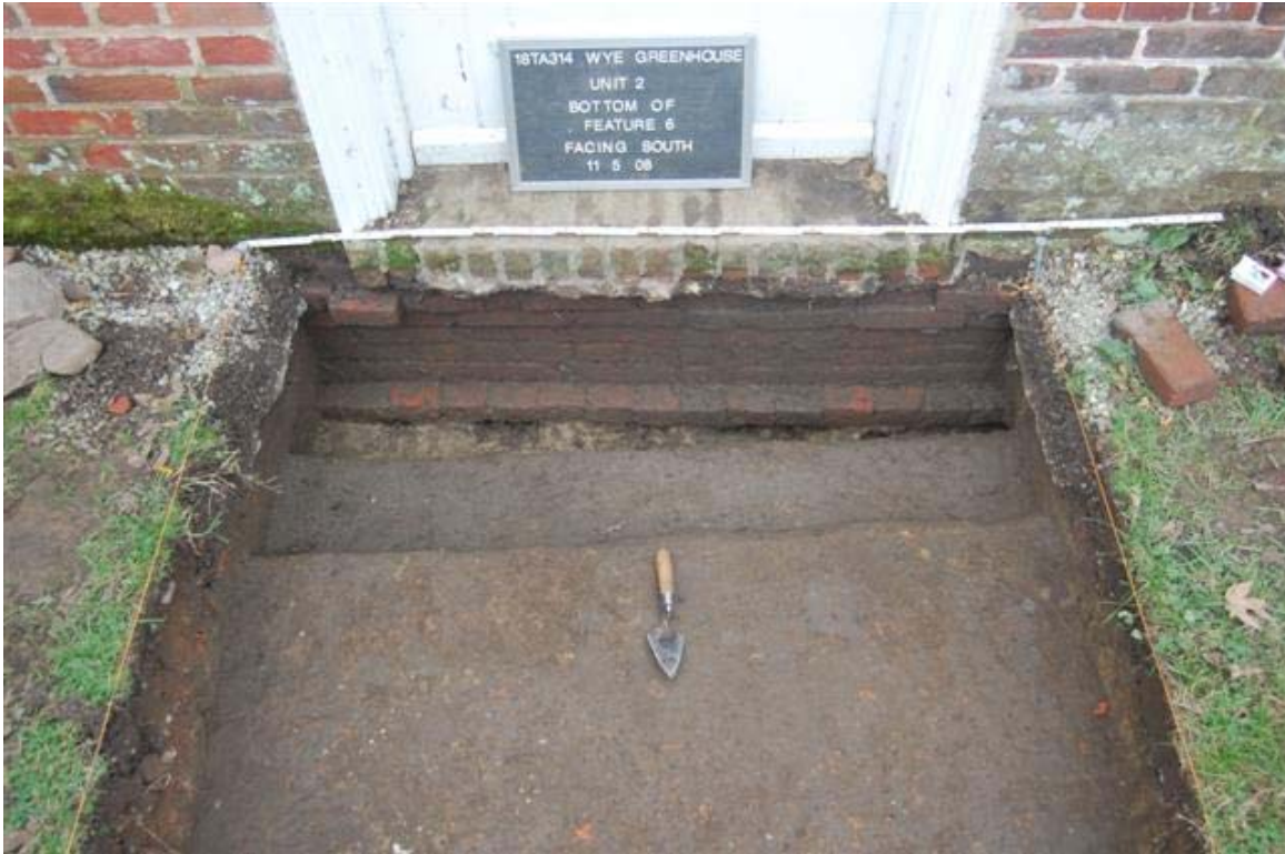
Figure 5.9 – Unit 2 Builder’s Trench (Feature 6) – The Builder’s Trench revealed a dry-laid foundation supporting the living quarter behind the main block of the greenhouse. The clay subsoil showed “pockets” or small voids, most likely due to rodent and root disturbance. Photo by Stephanie Duensing
