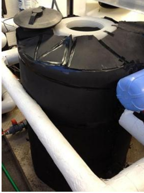
Figure 23: Cold water storage tank
