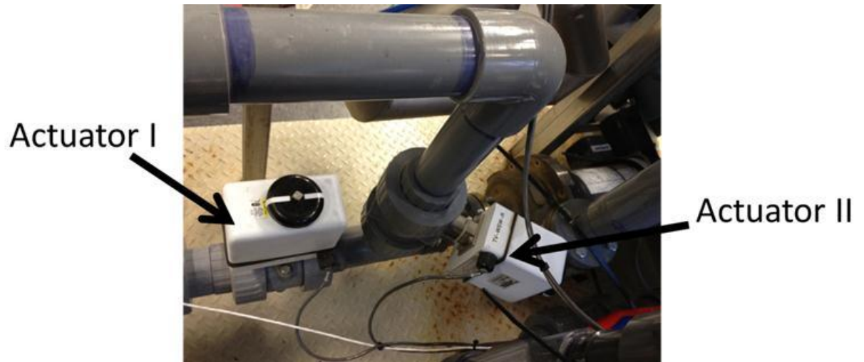
Figure 27: Actuator and valve for water temperature control
