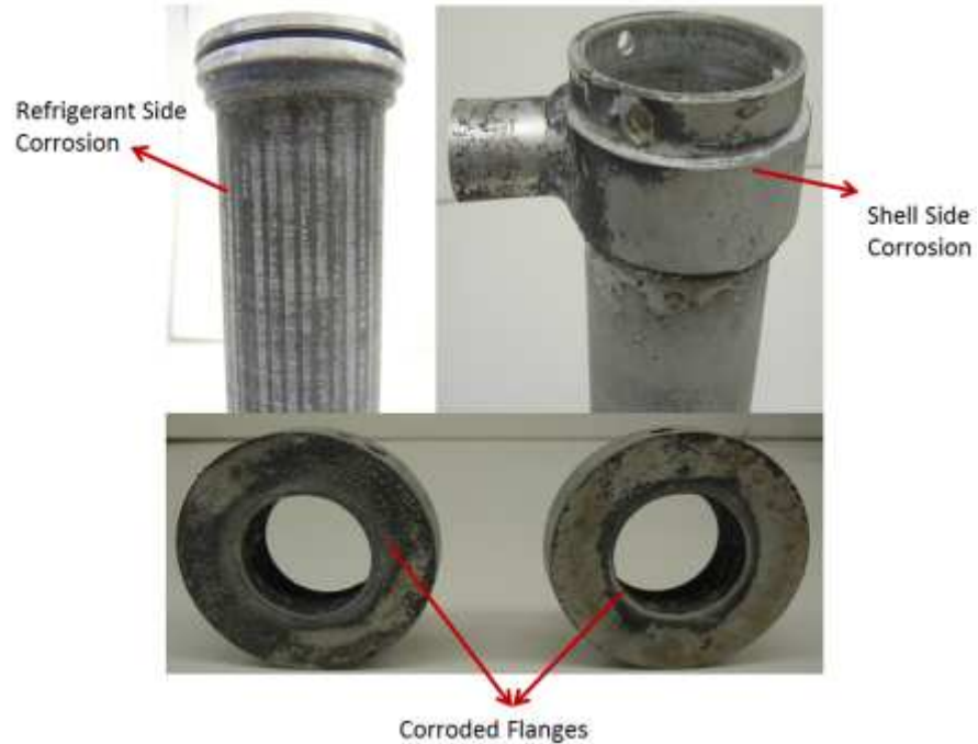
Figure 6-34: Corrosion from ammonia water solution at ammonia test facility
