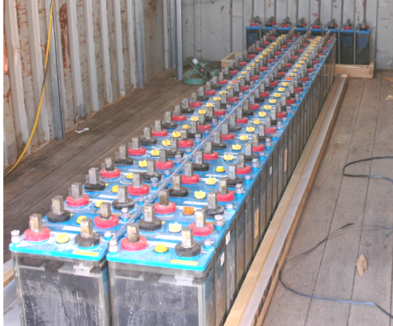
Figure 22. Photo of nominal 125Vdc battery bank used as power source in dc circuit testing. Photo is prior to terminal connection and located in climate controlled sea container.
