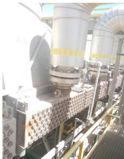
Figure 1. Air cooled heat exchanger (view from the front side)
