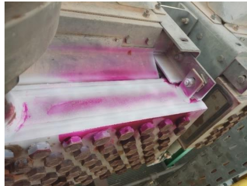
Figure 4. Results of PT testing of the weld joints
