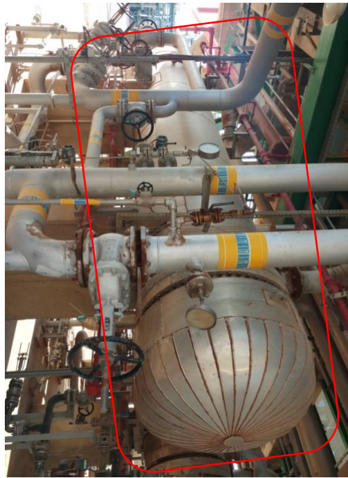
Figure 1. Oil-oil shell and tube heat exchanger
