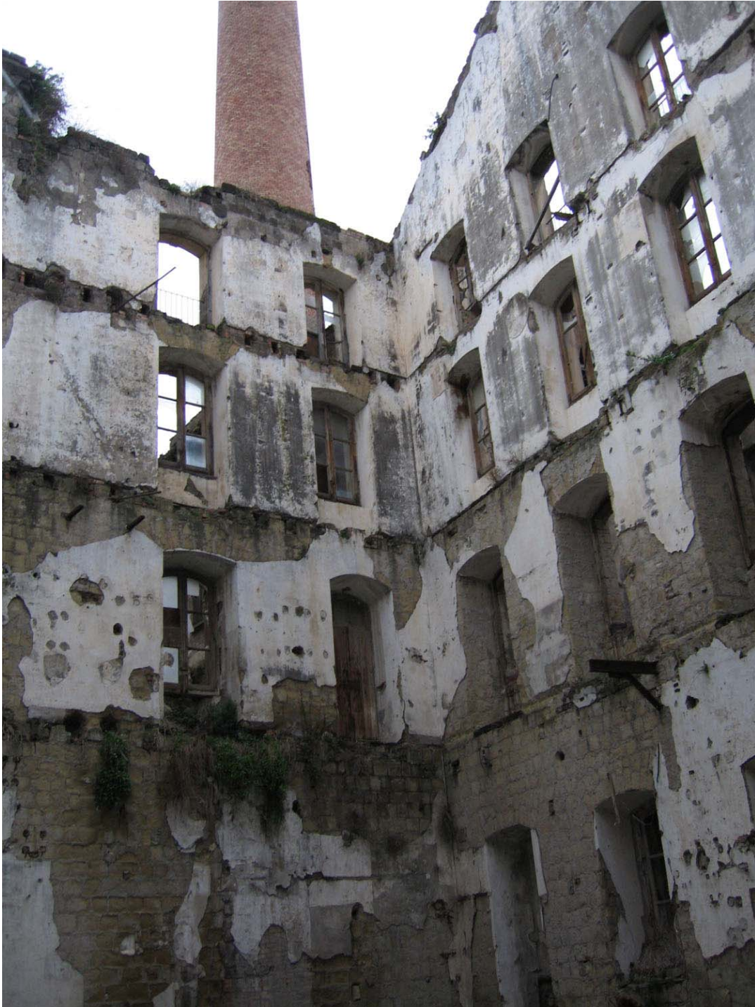
Figure 6-2-8. Interior elevation of historic building shell and the adjacency to historic smoke stack
