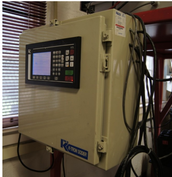
Figure 3.5 - KCM control system for K-TRON pellet feeder
