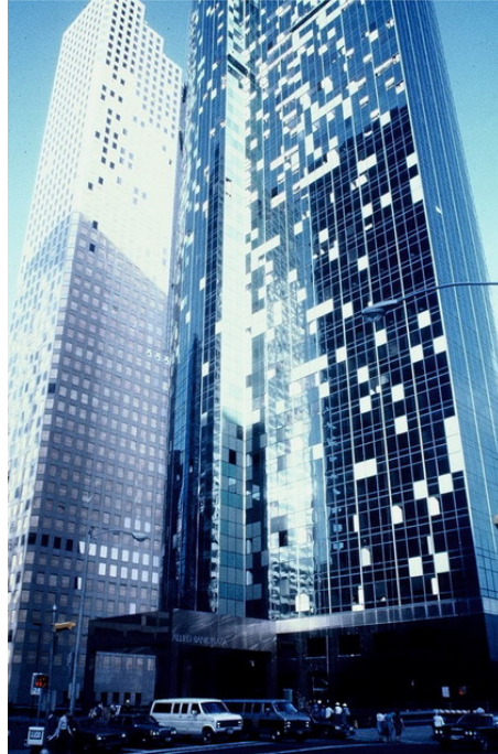
Figure 1.2: Façade Failure Due to Hurricane Alicia in 1983, Houston, TX (USACE 2010)
