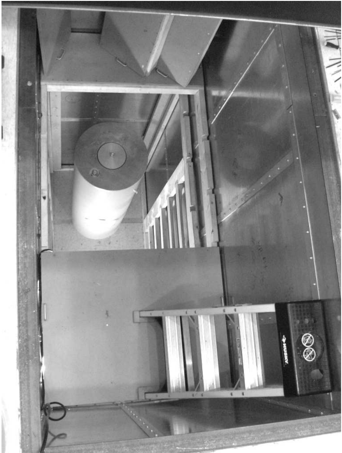
Figure 4.1: View into dewar pit showing construction of platform. Three panels of the platform floor have been removed, and stand on the panel in the back. Cross-beams of the platform panels fit into the notches in the scaffolding, at either of two heights. The dewar is stored below the platform. The ladder to the bottom of the pit (4m depth) is visible on one side. A stepladder leads to the top of the pit.
