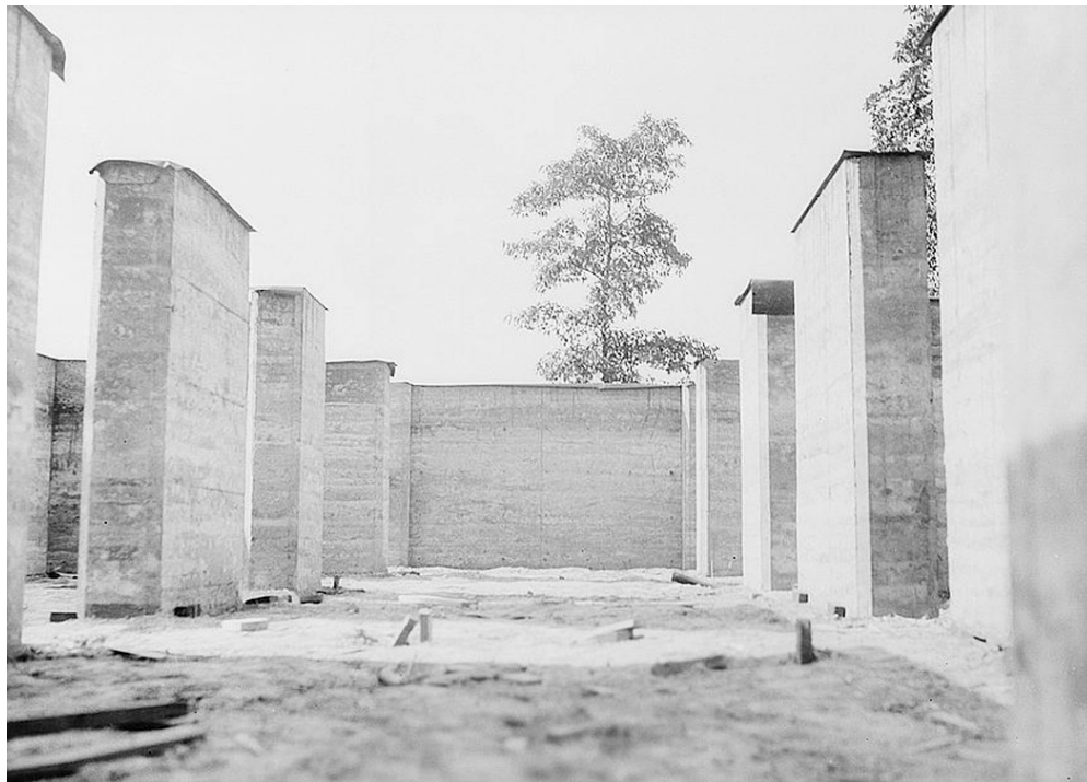
Figure 13. Completed rammed earth walls at Gardendale ( photograph from the Library of Congress, Prints and Photographs Division ).
