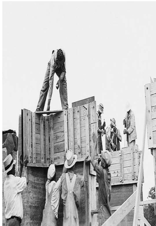
Figure 12. Workmen removing wooden shuttering from completed wall section (photographs from the Library of Congress, Prints and Photographs Division).
