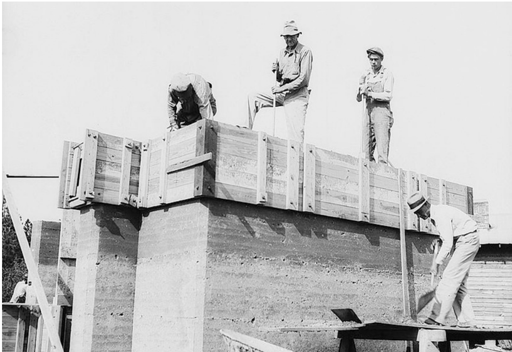
Figure 10. Workmen adding rammed earth layers to a wall at Gardendale (photographs from the Library of Congress, Prints and Photographs Division).
