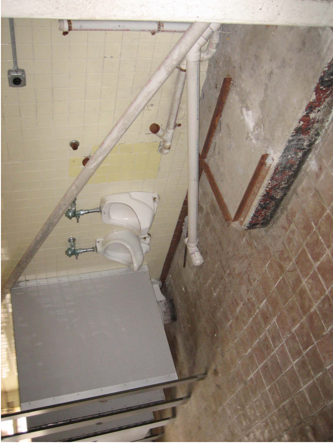
Figure 25: Deteriorating restroom facilities before renovation. Photo courtesy of Bruno Grinwis, BBGM architects, 2006.
