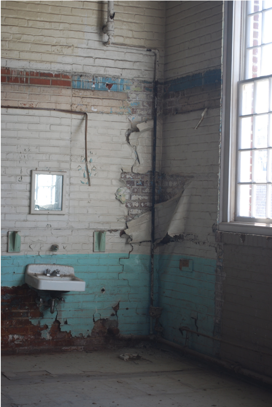
Figure 6: Stabilized but unrestored dormitory bathroom. Photo by author, 2009.
