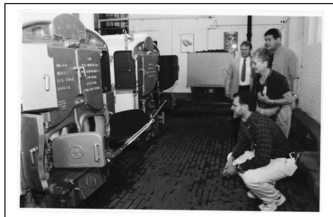
Boiler and furnace room. Photo Courtesy of the Preservation Society of Newport County.
