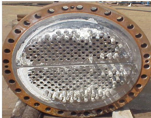
Figure 1: Scale formation at the inlet of a tube bundle [10]
