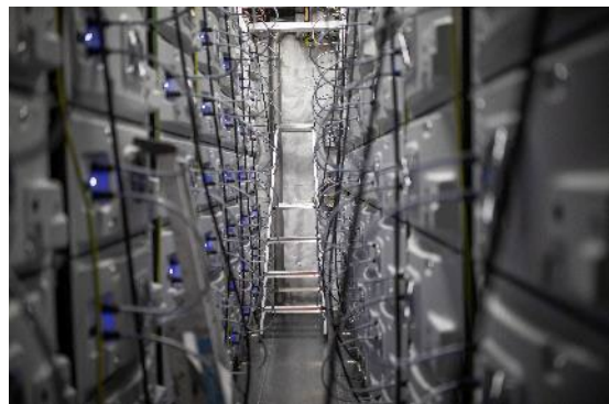
Fig. 20, Typical string of Corvus Dolphin Power batteries
