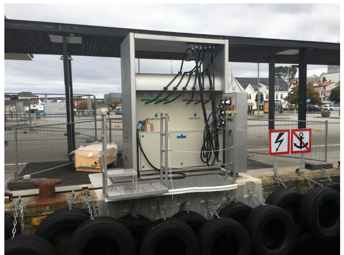
Fig. 23, Charging point for the Stavanger Demonstrator at Fiskepiren, Stavanger (6 plug-ins)
