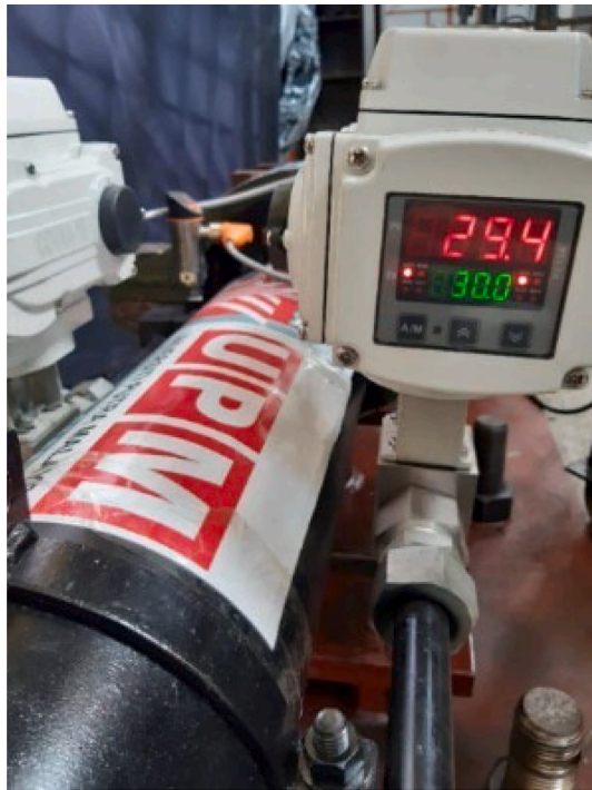
Fig. 11. Valve Screen, the command from PLC panel (Greenlight), valve feedback (Red light). (For interpretation of the references to colour in this figure legend, the reader is referred to the web version of this article.)
