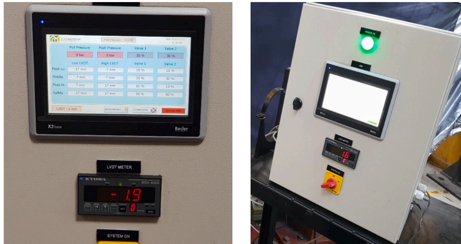
Fig. 13. Setup of the PLC controller.
