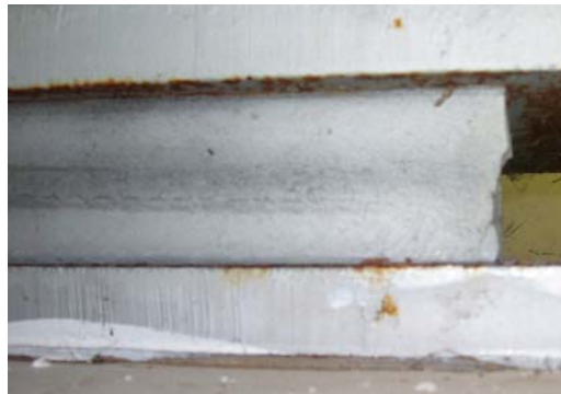
Figure 3.1 - Pad Deterioration in Bridge #1169
