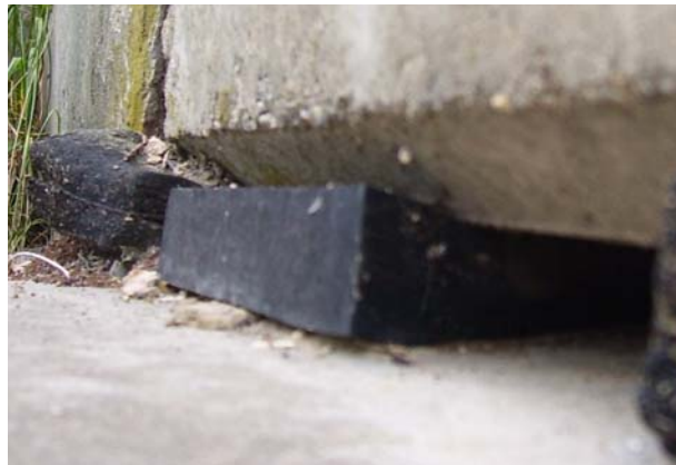
Figure 3.10 - Crushing in a Slab Bridge
