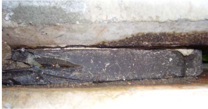
Figure 3.9 - Deterioration Due to Poor Quality
