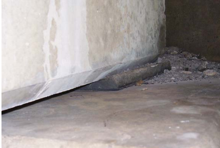
Figure 6.1 – Bearing Creep in Bridge 1097
