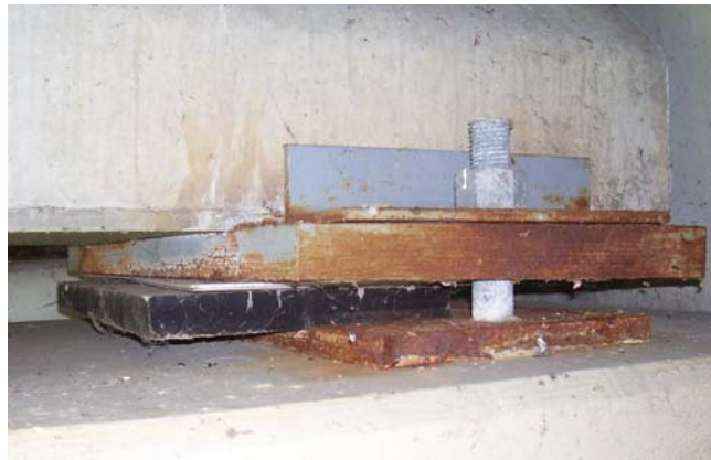
Figure 3.2 - Bearing Slip in Bridge #9015
