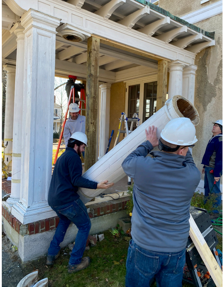
Porch restoration at the First Amendment Museum, Augusta, ME. Photo: Maine Preservation.
