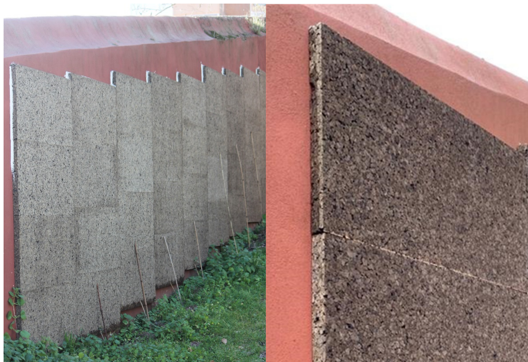
Figure 2. Expanded cork boards used to build the indirect green façade, disposed of in an outer wall of Ajuda Botanical Garden ((left panel), the whole set; (right panel), detail of the cork boards).
