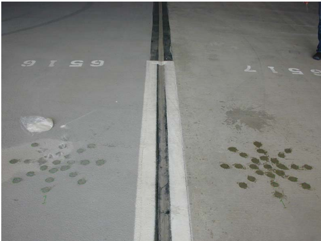
Figure 6.2 Locations of test measurements; the concrete surface is covered by a membrane on the left side of the expansion joint.
