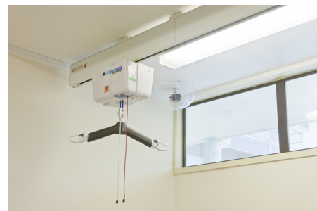
Ceiling tracking with hoist
