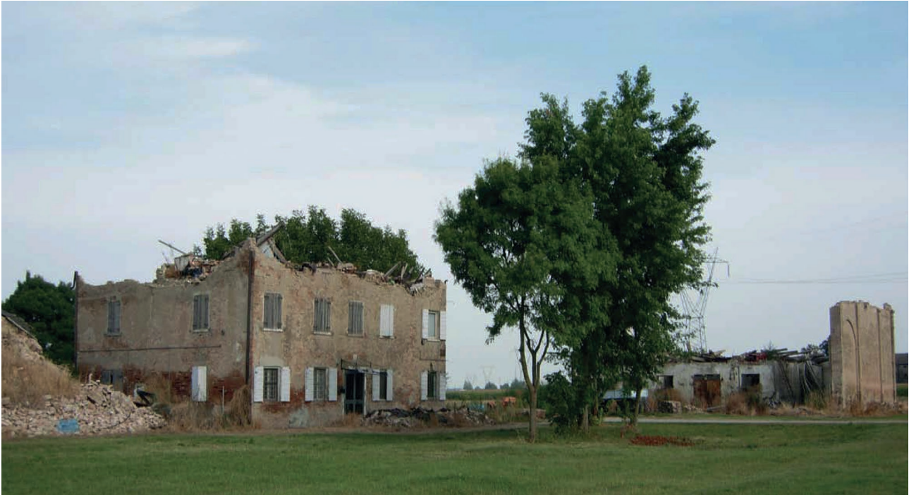
Figure 1 | San Giacomo Roncole in the district of Mirandola, Modena. In the historic courtyard, the stable-barn and the dwelling collapsed due to wall-roof interaction.
