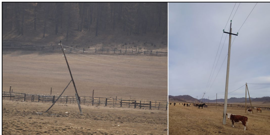
Fig. 6. Electric pole of line No. 18 in emergency state and a herd of cows and horses grazing in the close vicinity. Photos by E. Shnyder.
