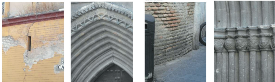
Figure 9. a y b) fractures; c) moist area; d) erosion and black crust
