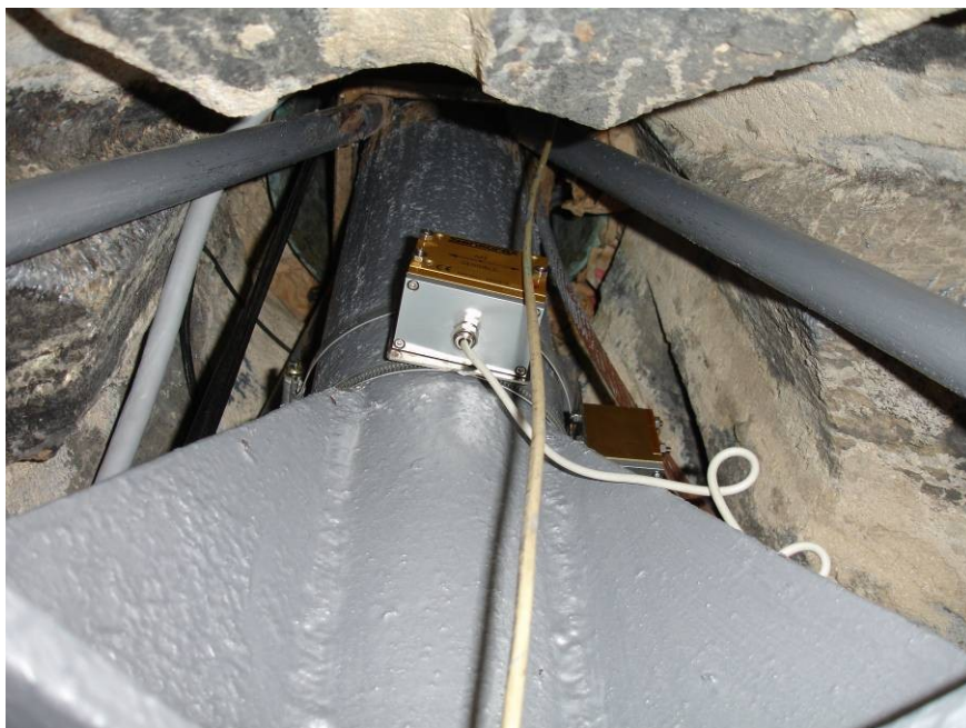
Figure 7. Mounting of inclinometers inside the dome of the Giralda Tower (referred to as section 0 in Figure 4.).
