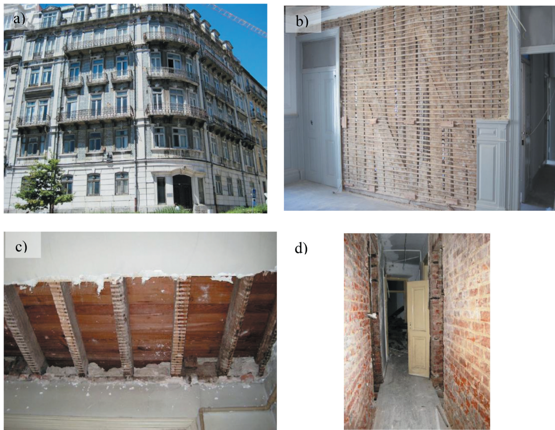
Figure 7. “Gaioleiro” typology: (a) aesthetic of the building; (b) “tabique” partition walls; (c) timber floor supported on the adulterated “frontal” walls or brick masonry; (d) brick masonry interior walls.
