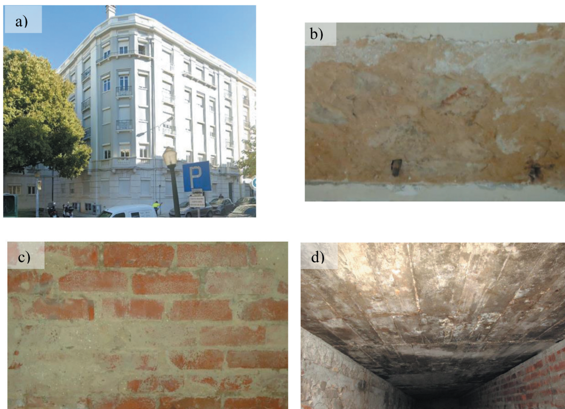
Figure 8. “Placa” typology: (a) aesthetic of the building; (b) rubble stone masonry wall; (c) brick masonry wall; (d) concrete slab simple supported on the masonry walls.
