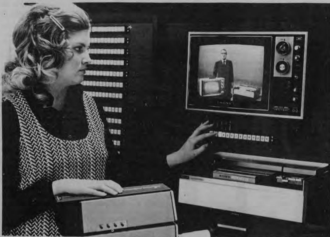
Senior education major, Mrs. Pete Vasquez Jr., demonstrates the ease of operation of the newly installed electronic educational instruction system in the education building at Pan American University. From this control console, Mrs. Vasquez can send any of 14 audio or video programs to 16 different mobile teaching stations in the building.
