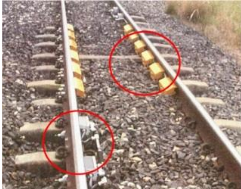
Figure 1: WILD System, Wheel Sensor (Left circle) and Accelerometers Installed on Track (Right Circle) [7]
