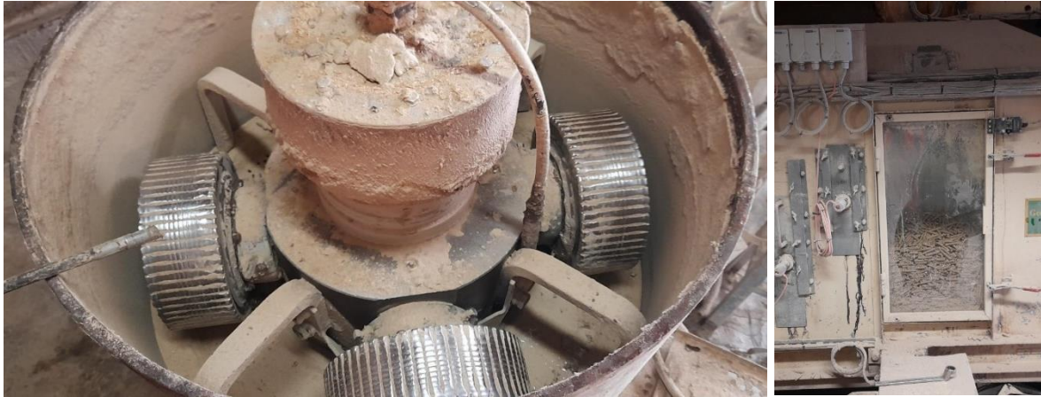
Figure 4: Roll presses of Boortmalt's pellet production.
