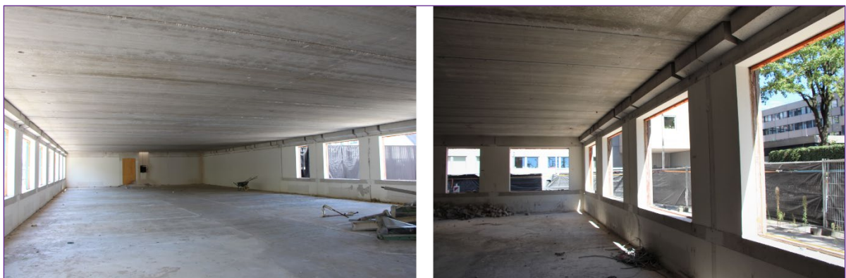
Figure 18. The Dutch donor building. All the finishes have been removed, only the structure of the building is visible and can be scanned
