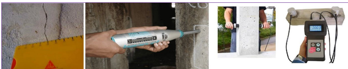
Figure 19. In-situ testing from left to right: crack width measurement, Schmidt hammer testing and cover depth measurement.
