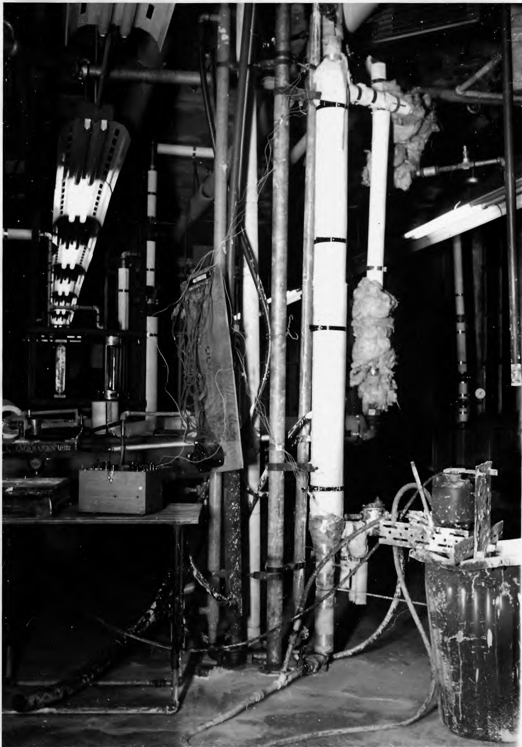
Figure 2a View of apparatus showing heat exchanger, coolers, potentiometer, multipoint thermocouple switch, and slurry storage tank with submerged circulating pump.
