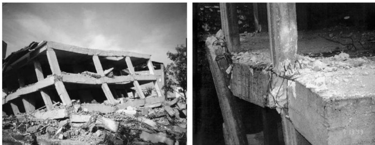
Figure 1. The collapse of the concrete building at the earthquake of Kocaeli in 1999: (a) Joint failure at the collapsed building; (b) Brittle failure of concrete joint [3]
