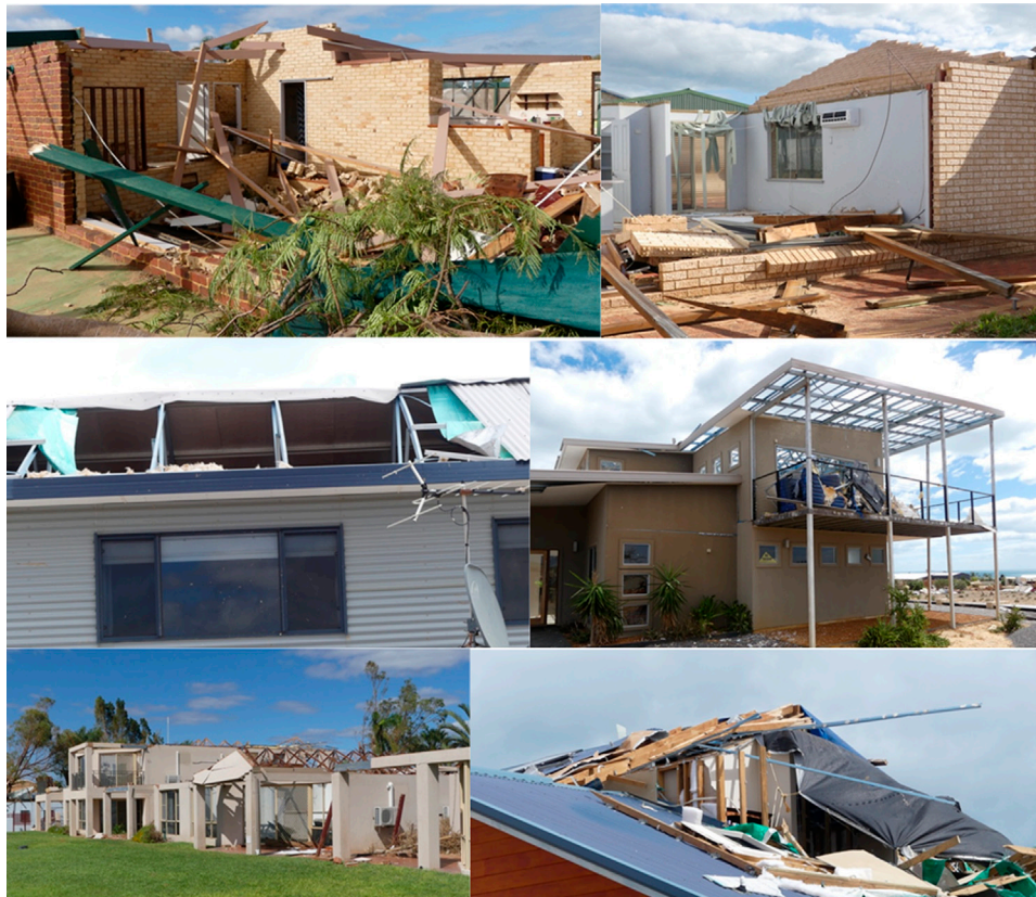
FIGURE 5 Roof damage because of high internal pressure.
