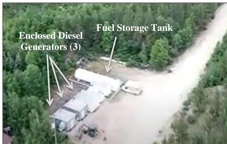
Figure 4-2: Aerial photograph of the CCM generation assets located in Kinoosao, Saskatchewan. SaskPower has two rate categories for residential electricity service, a standard rate and a rate for residences served by diesel generators. Household bills include three parameters, a basic monthly charge, an energy charge and a federal carbon charge. Electricity rates start at $32.90 per residence per month. CCM households pay $0.14 for their first 650 kWh/month of electricity consumption and $0.53 per kWh/month after that. The rate that all households pay for the
