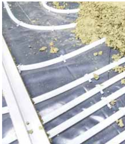
Grant's Uflex underfloor heating system.
