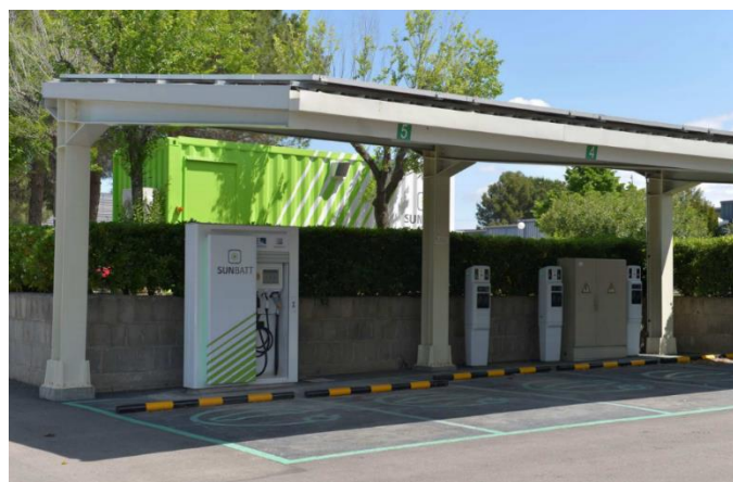
Figure 13: SUNBATT EV Charging station [26]
