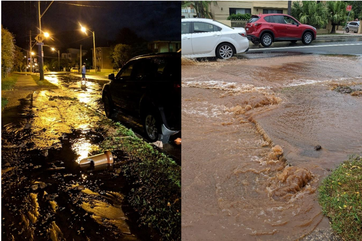
Figure 3.12: A burst mains water pipeline outside my apartment in Wollongong in October 2018 (left) and again in January 2020 (right). Source: author.
