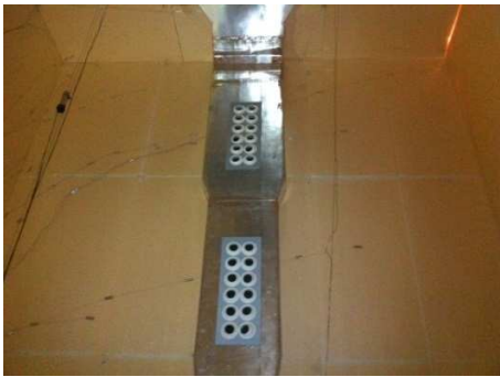
Figure 4. HVAC system. Air distribution system
