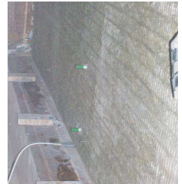
Hot wire anemometers to measure the air chamber air velocities in the central vertical axis in two different levels.
