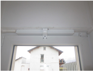
Automatism for windows opening/closing.
