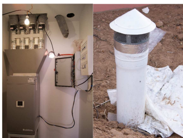
Heat Pump and Ground heat exchanger
