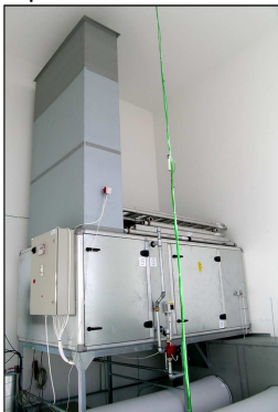
Ventilation system in the experiment room
