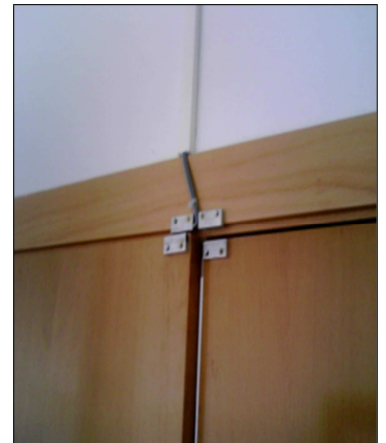
Magnetic switches to detect if doors are closed or not closed
