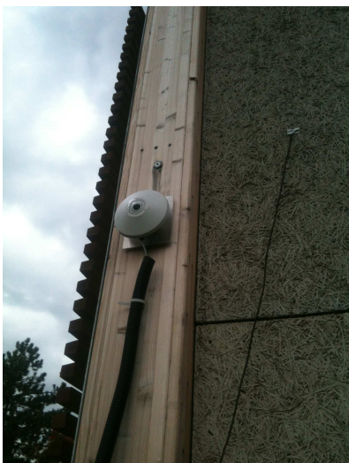
The pyranometer device to measure the global vertical solar radiation on test wall.
