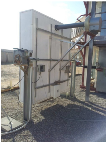
Front and rear views of the Test Reference Environment of Lleida (TRE-L) at the LOTCE center [3].
