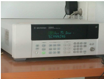
HP Agilent 34980A data acquisition system for logging and controlling the PASLINK tests.
