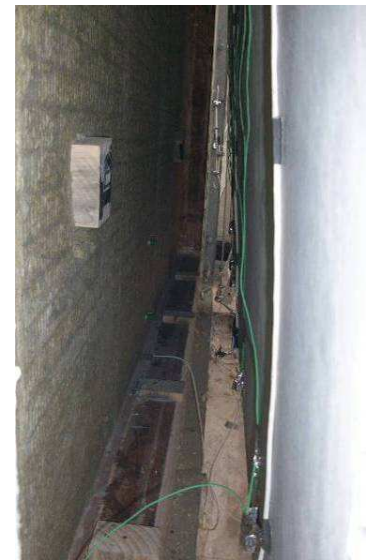
Closing the air chamber, wooden separators to maintain the air gap uniform. Thermopile cables in green.
