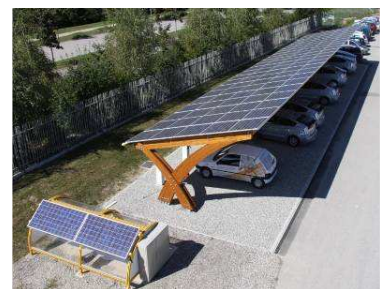
Electrical cars and solar station.
