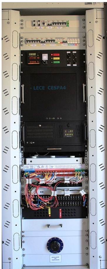
Data Acquisition and Control System
