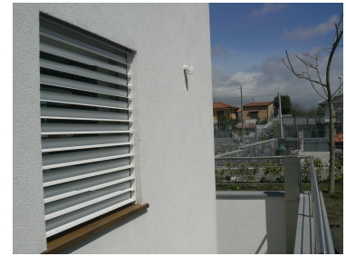
External movable solar shading blinds, automatic controlled. The actual position of them will be logged at each time step.
