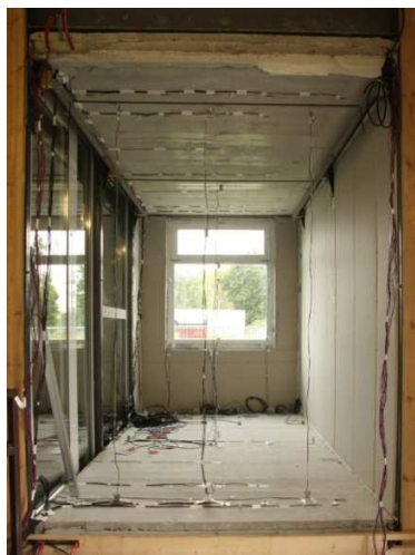
Full scale test room during construction: concrete floor and ceiling, window in SW façade, windows in room side wall
