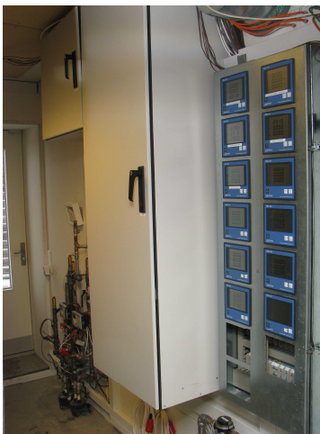
Heat meters at EnergyFlexLab.
