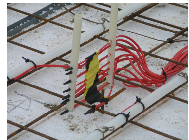
Embedded temperature sensors in the floor of one of the side-by-side test rooms in EnergyFlexLab before concrete was poured in.
