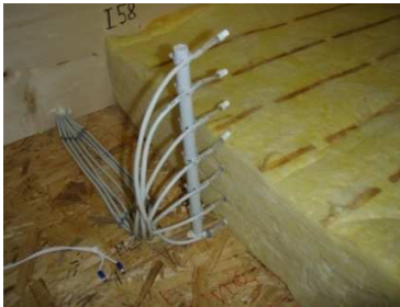
Combined heat/moisture sensors in roof assembly
