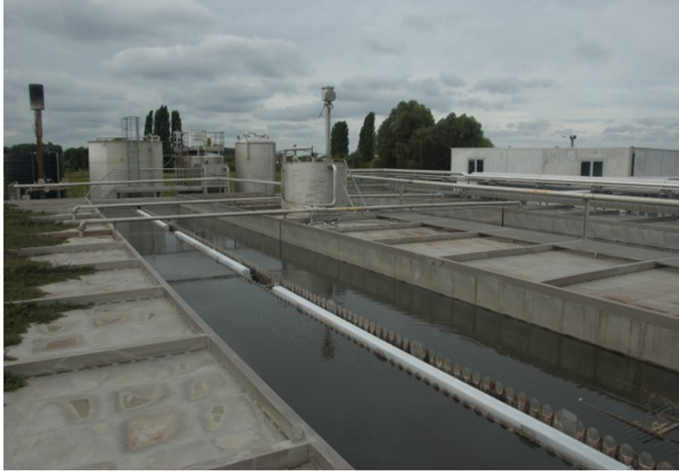
Figure X-5. A partial view on the wastewater treatment plant of the potato factory Agristo, Harelbeke, Belgium. The digestate originating from the anaerobic digestion process is pumped into a gutter system for further processing. The basin has a depth of less than a meter and the effluent is constantly in motion.
