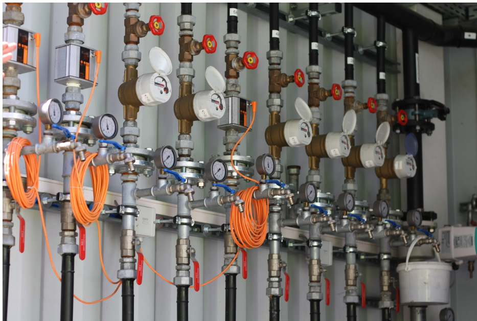
Flow regulators, soil remediation plant, Geneva
