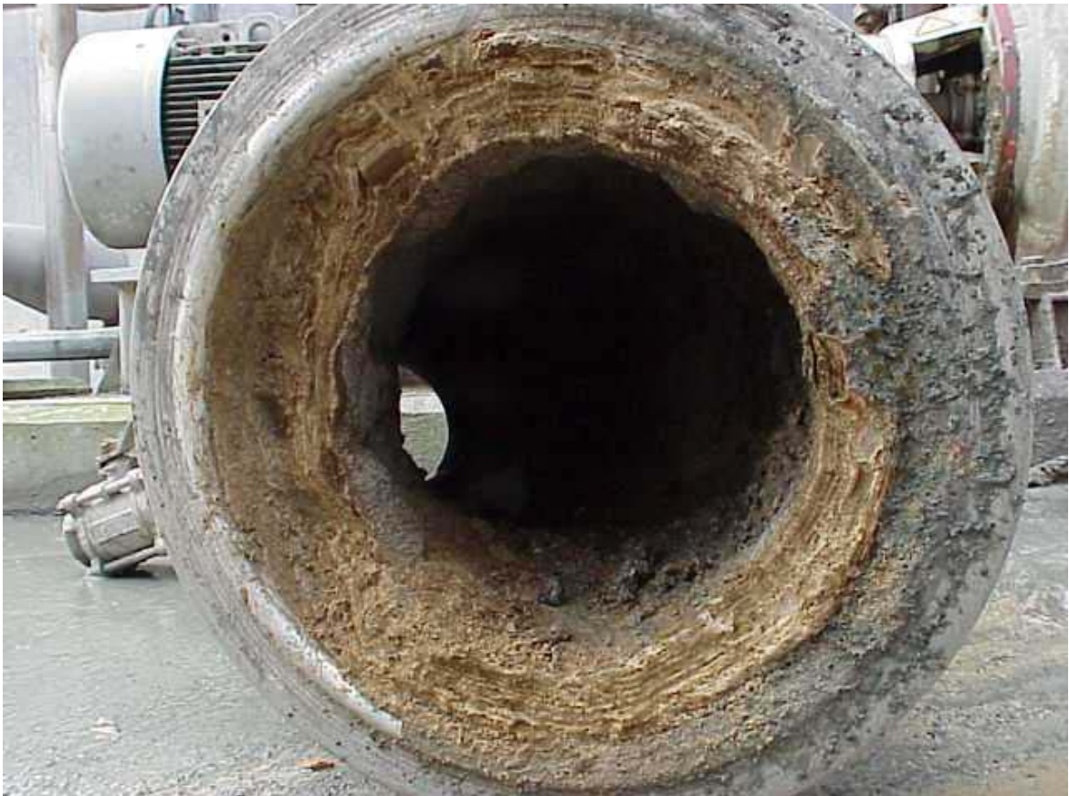
Figure 8.2. CaCO 3 scaling-damage on a concrete pipeline which is part of downstream processing of calcium-rich wastewater from a paper-recycling facility.
